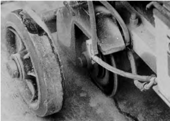
Figure 9.1. Random crack saw
