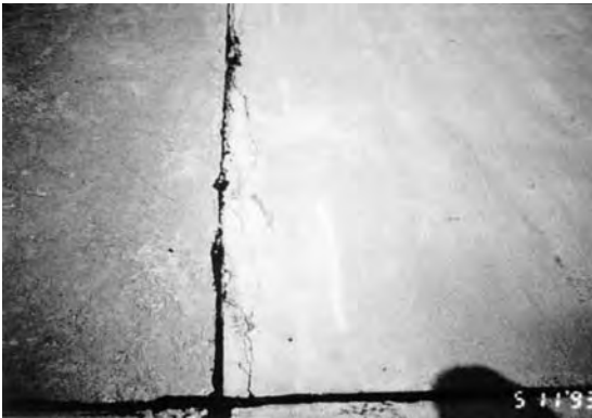
Figure 4.1. Moderate-severity spalling along an expansion joint
