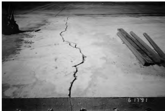
Figure 10.2. A freshly sawed crack
