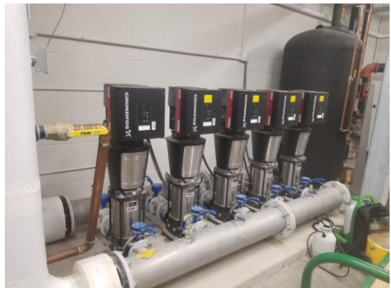
Ground loop pumps
