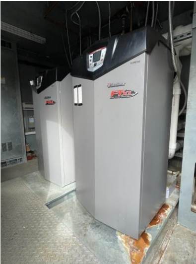
Natural gas-fired boilers
