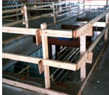
Properly installed guardrail system.
