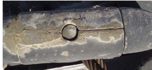
Figure 2-28 Missing Lead Plug
