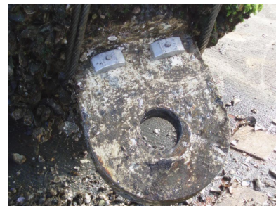
Figure 2-51 Chain Stud Anode on Buoy Tension Bar
