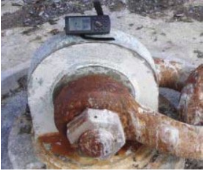
Figure 3-27 Minimal Corrosion on Tension Bar Padeye
