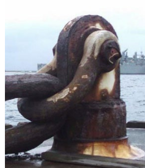
Figure 3-28 Excessive Corrosion on Tension Bar Padeye
