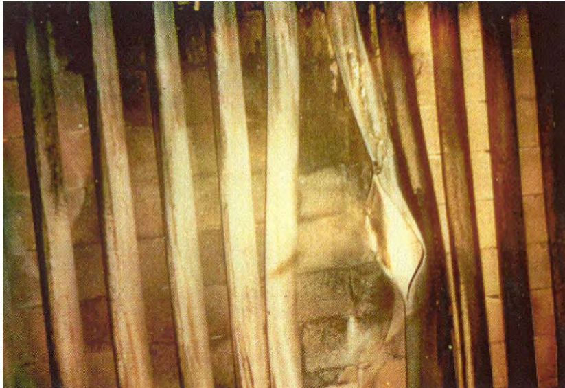
Figure 4-9 Failed Boiler Tube
