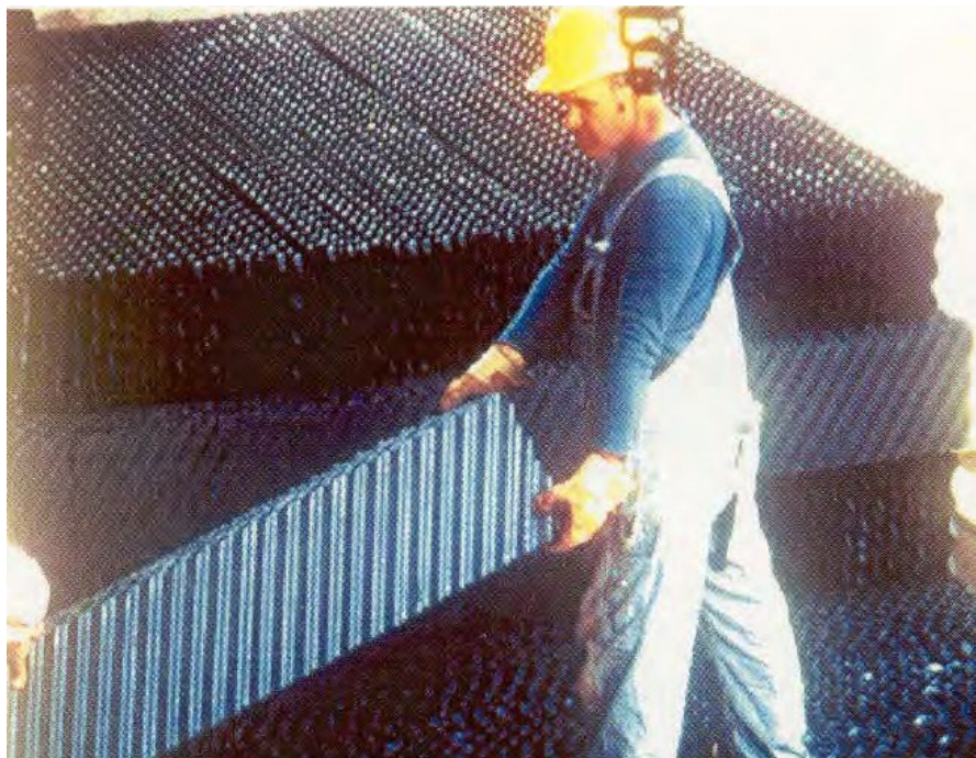
Figure 5-11 High-Efficiency Cooling Tower Film Fill
