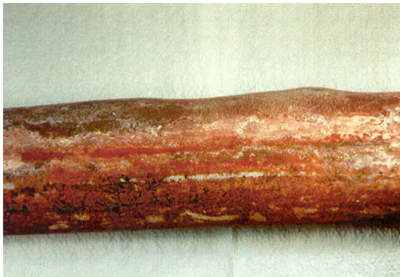
Figure 4-8 Metal Fatigue on Boiler Tube
