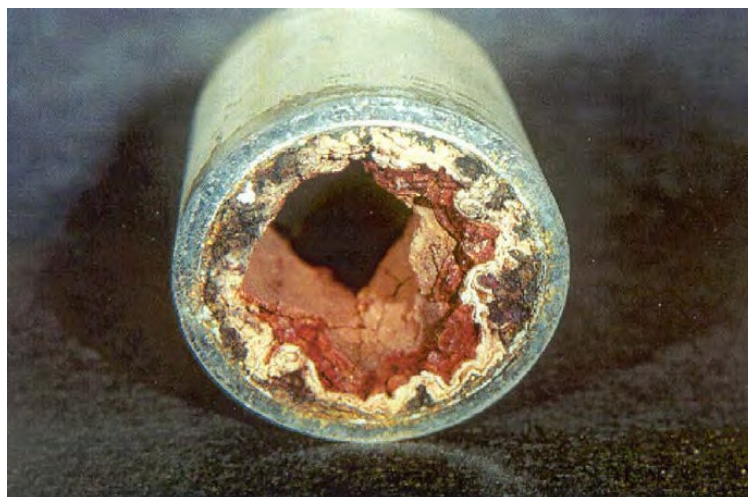
Figure 4-5 Scaled Boiler Tube
