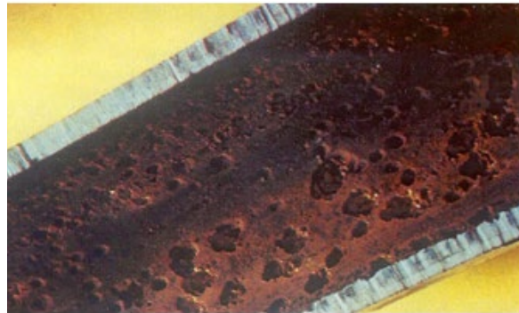
Figure 4-4 Boiler Tube Oxygen Pitting
