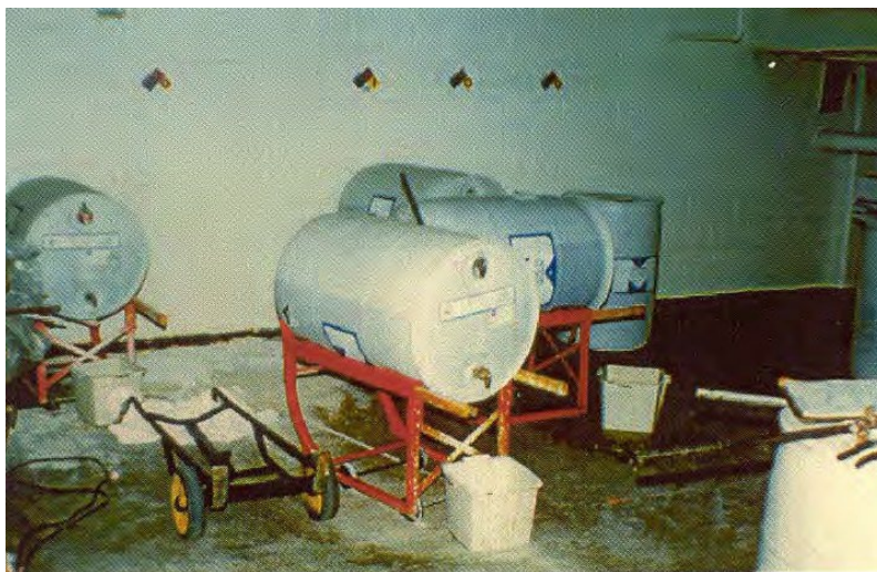
Figure 8-2 Manual Chemical Feed System
