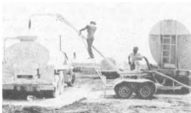
Figure 4-30. Jet slurry mixing plant.
