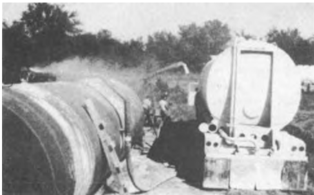
Figure 4-29. Slurry mixing tank using recirculating pump for mixing hydrate and water.
