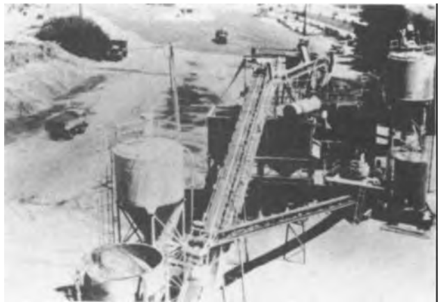
Figure 4-22. Enclosed soil holds lime for adding to marginal crushed stone base material.
