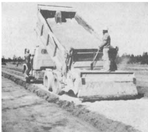
Figure 4-8. Mechanical cement spreader attached to a job dump truck spreading cement in regulated quantities.
