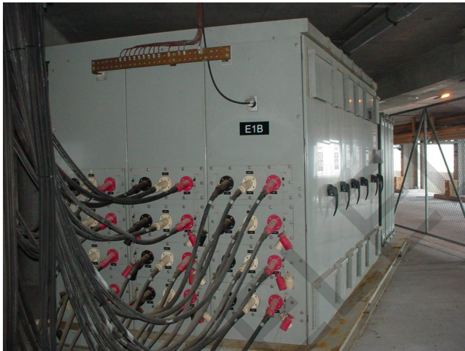
Figure 12-6. Double-Deck Pier Switchgear
