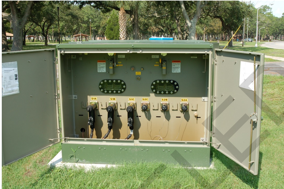
Figure D-3 Cooper VFI Switchgear
