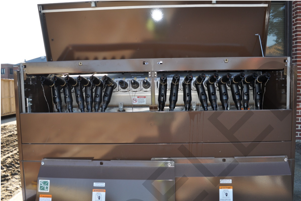
Figure D-1 S&C Vista Switchgear
