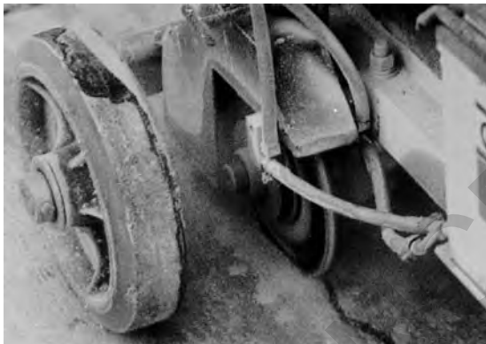
Figure 9.1. Random crack saw
