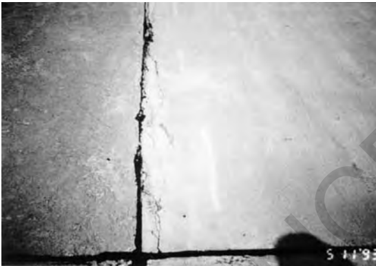
Figure 4.1. Moderate-severity spalling along an expansion joint
