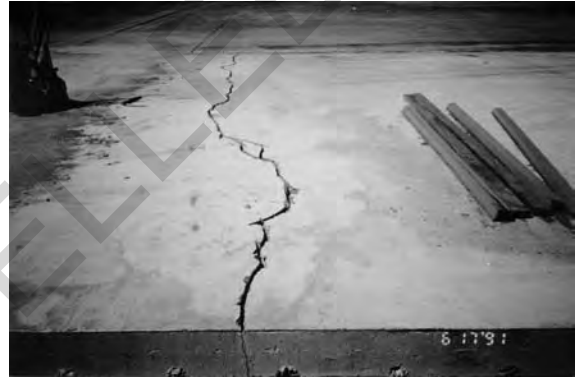
Figure 10.2. A freshly sawed crack
