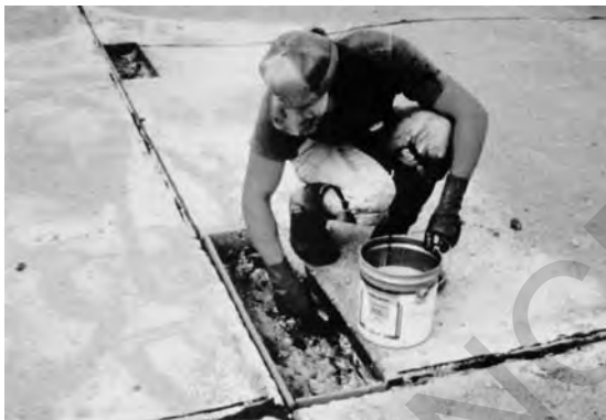
Figure 16.1. Application of bonding agent to the concrete surface. Note the joint filler bordering the repair area
