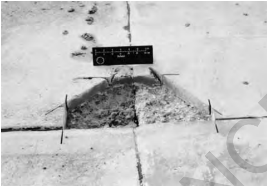
Figure 15.1. A spalled area on both sides of an expansion joint ready for installation of joint filler
