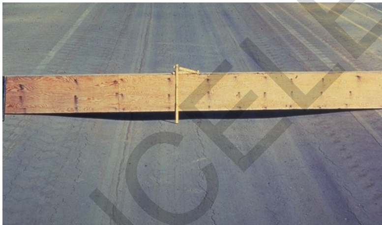
Figure 3-8 Rutting of the Pavement Structure
