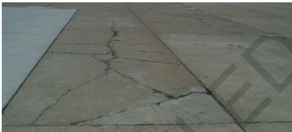
Figure 3-12 Shattered Slabs on Concrete Pavement
