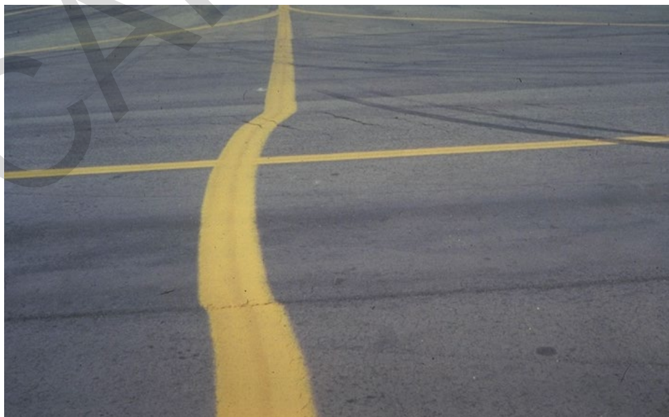
Figure 3-10 Slippage due to Loss of Bond
