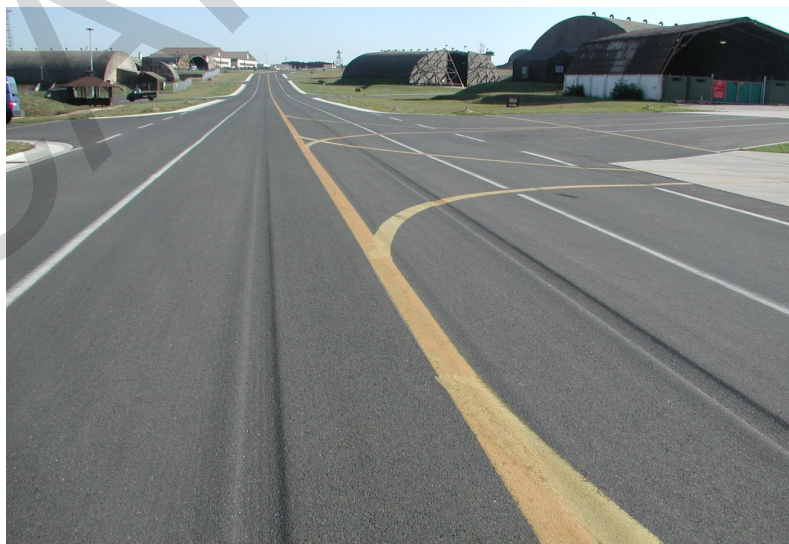
Figure 3-9 Rutting in the HMA Layers
