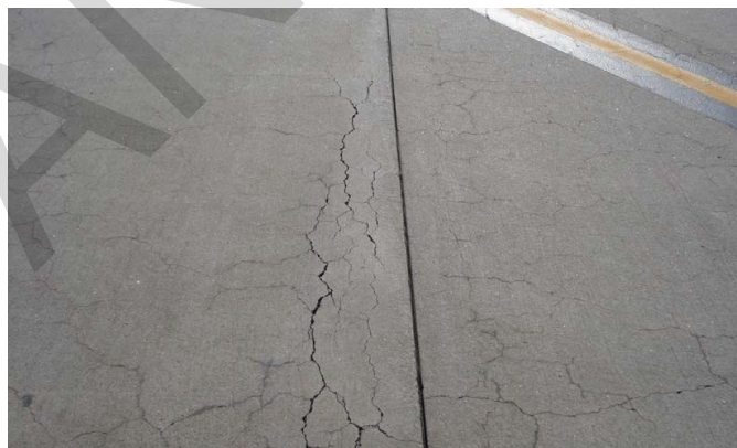
Figure 3-11 ASR Distress (Scaling/Map Cracking) on Concrete Pavement
