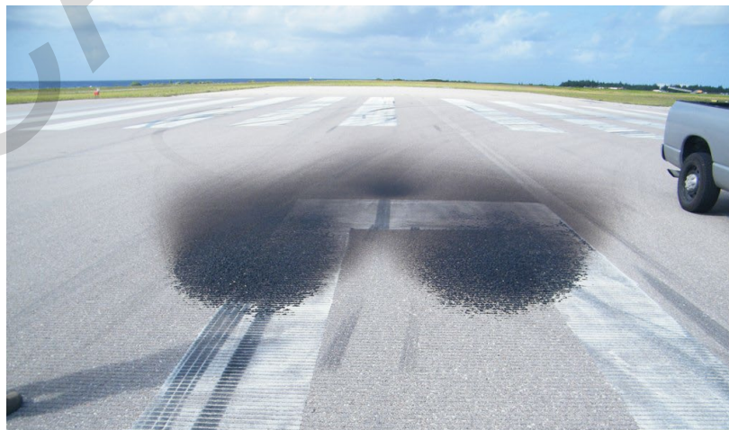
Figure 3-2 Jet Blast Damage
