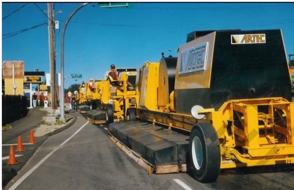
Figure 5-7 Surface Recycling Heating Unit
