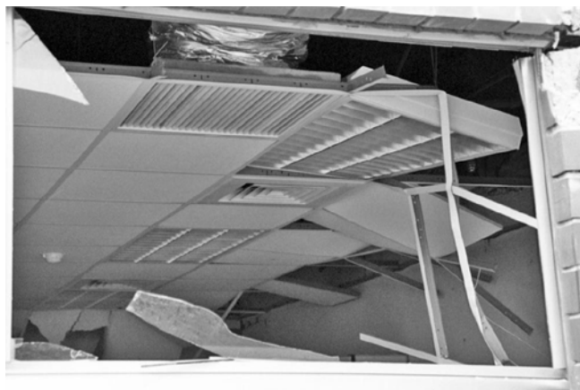
FIGURE C13.1-4 Damaged Ceiling System
