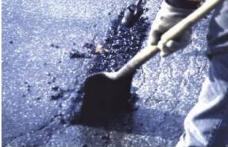
Figure 5. Pot hole filled with cold-patch.
