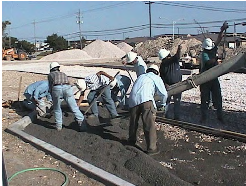
Figure A-3. Contractors installing the Ecocrete porous concrete system at Fort Hood.
