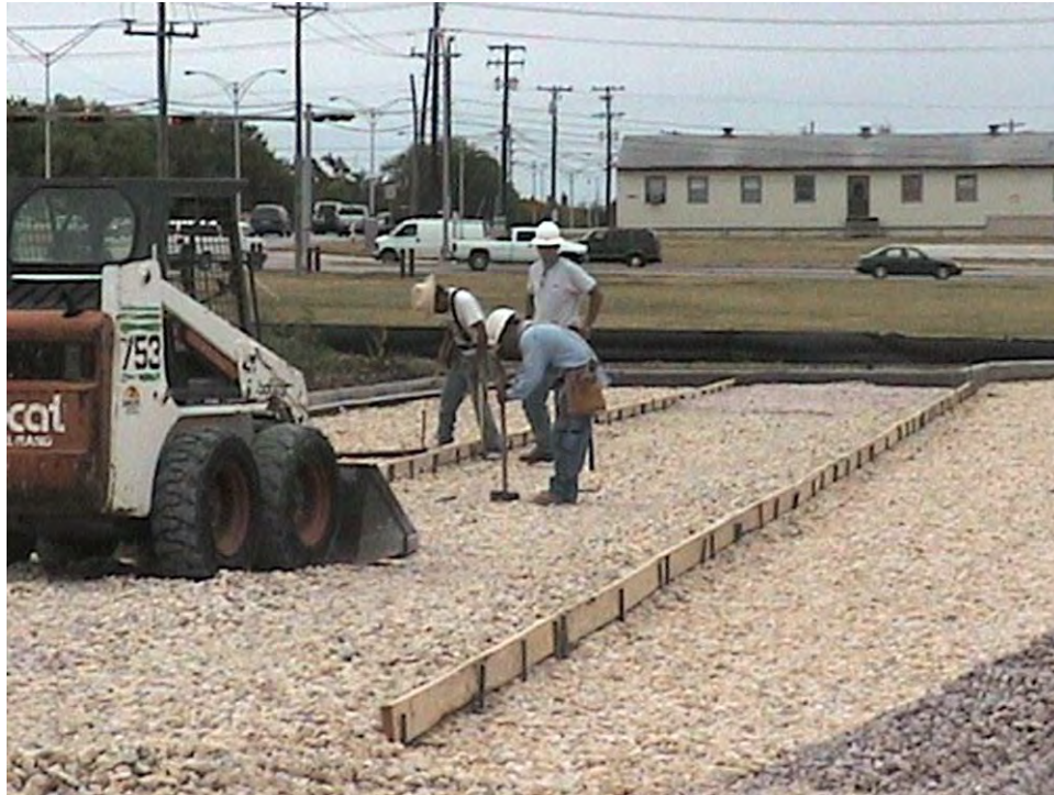
Figure A-2. Workers installing a 1 ½-in. layer of rock for the porous concrete system subsurface.
