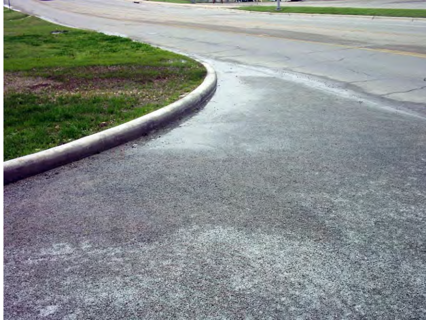
Figure A-8. Water seeping from the southeast end of the parking lot.
