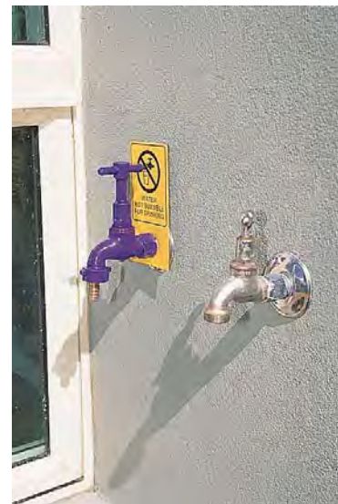
Figure 6. Separate faucets for potable and nonpotable graywater.
