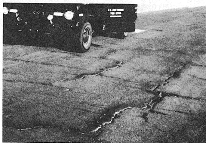
Figure B-14. High-severity block cracking.
