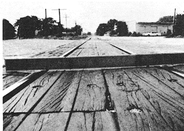
Figure B-53. Low-severity railroad crossing.
