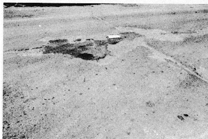
Figure B-129. High-severity scaling/map cracking/crazing.
