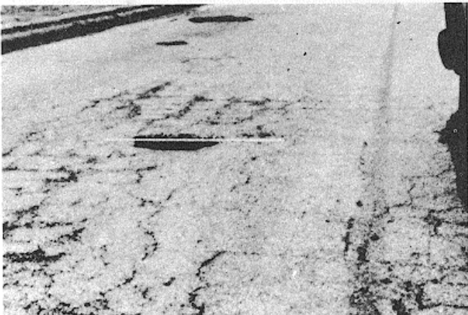
Figure B-50. Medium-severity pothole.
