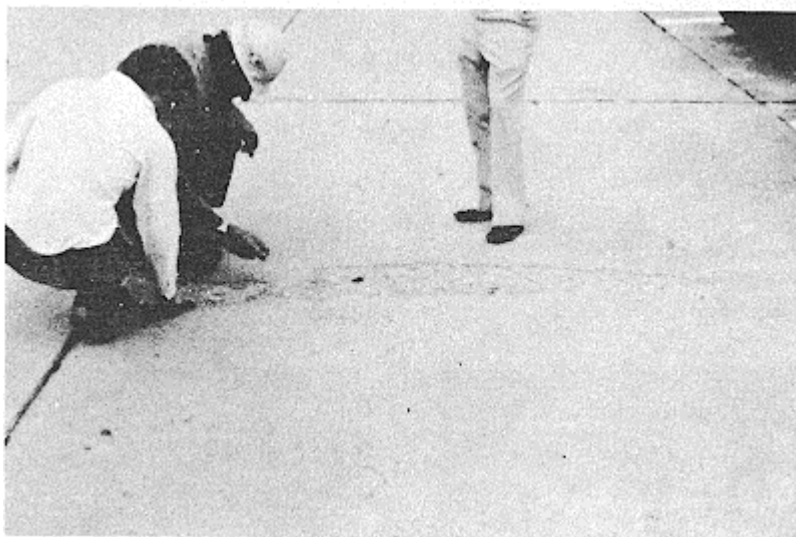
Figure B-87. Medium-severity durability cracking.
