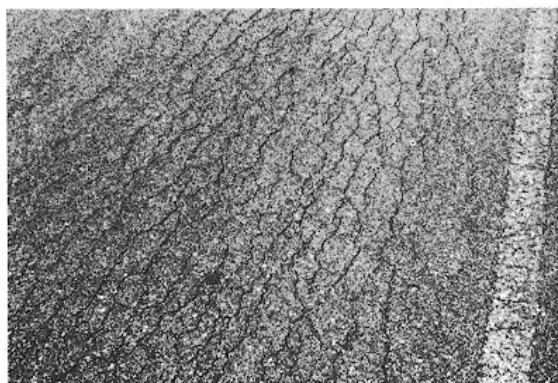
Figure B-5. Medium-severity alligator cracking.
