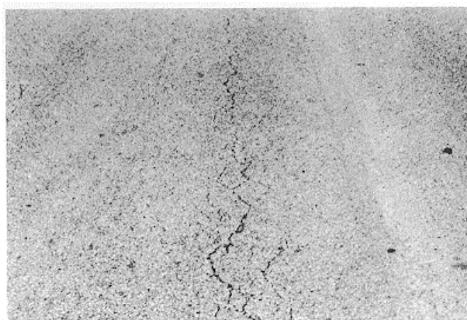
Figure B-2. Low-severity alligator cracking.
