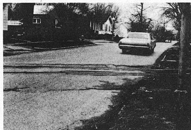
Figure B-55. High-severity railroad crossing.
