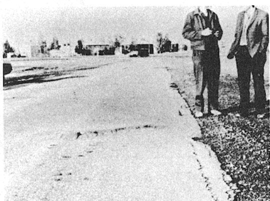
Figure B-16. Medium-severity bumps and sags.
