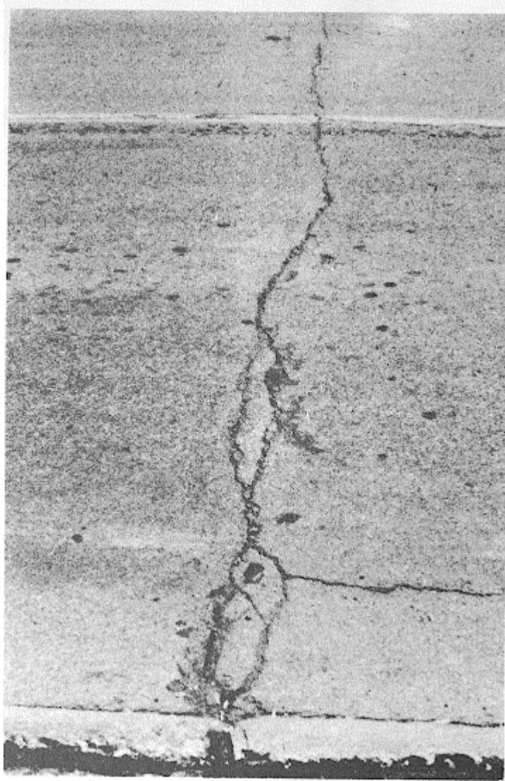
Figure B-32. Medium-severity joint reflection cracking.
