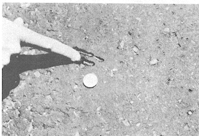
Figure B-9. Medium-severity bleeding.
