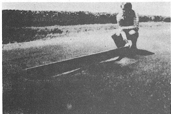
Figure B-23. High-severity corrugation.
