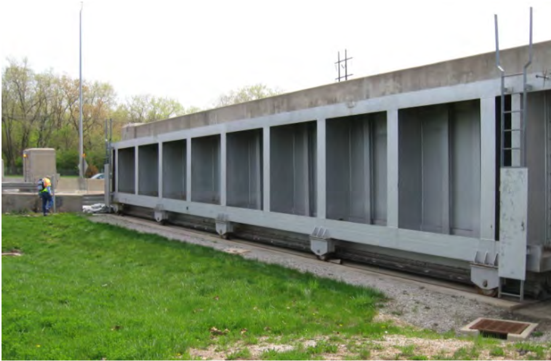
Figure F-5. Rolling Gate Closure Structure.
