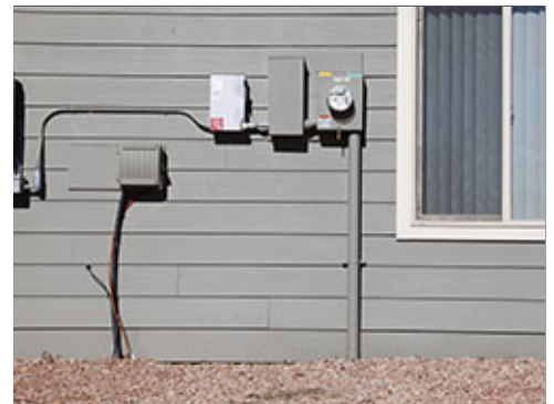
Components Painted to Match Wall
