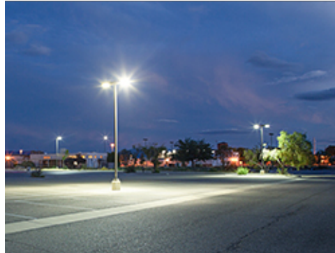
Parking Lot Pole Lighting with LED luminaires
