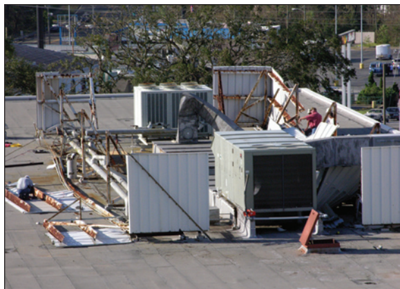
Figure 9. Several of the equipment screen panels were blown away. Loose panels can break glazing and puncture roof membranes.
