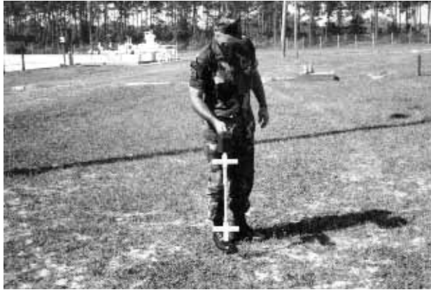
Figure 2.1. Using Induction Method to Locate Anodes.
