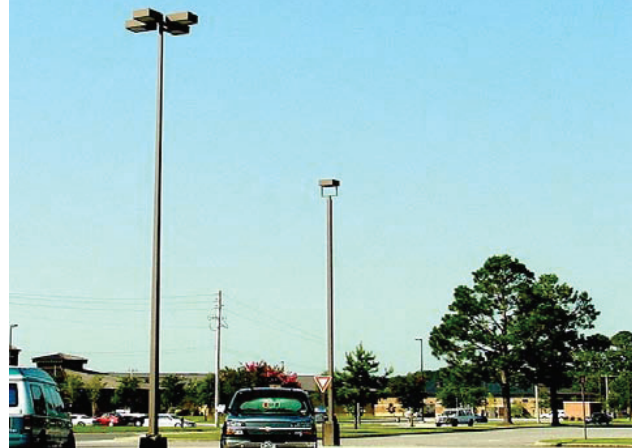
2-3p Parking and Area Lighting Fixtures.
