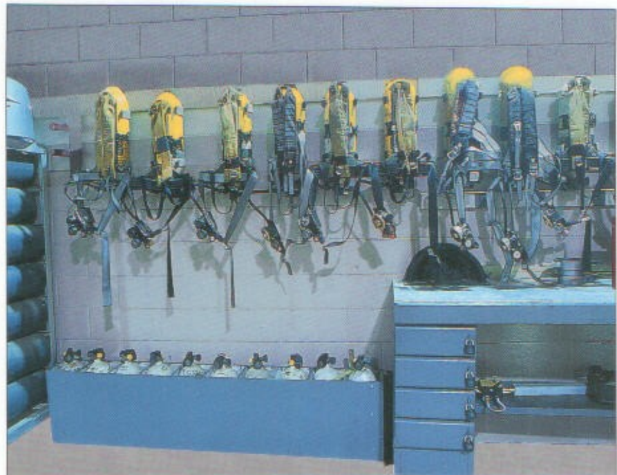
Design the SCBA maintenance and repair area to store 6-10 sets of apparatus, along with a mask pressure checking machine.
