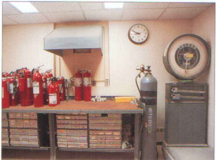
Fire extinguisher repair space should include a work bench, safety cage, spare parts bin, and dry chemical extinguisher recharge kit.
