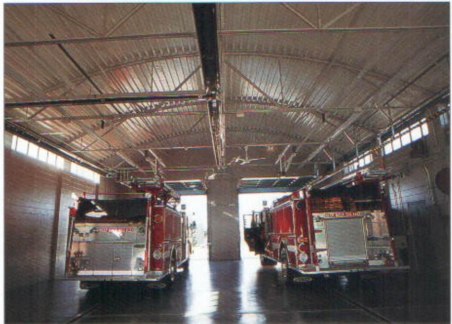
Place a trench drain parallel to the centerline of each vehicle. All apparatus room drains should have a fine grate cover and be connected to an approved oil/water separator.
