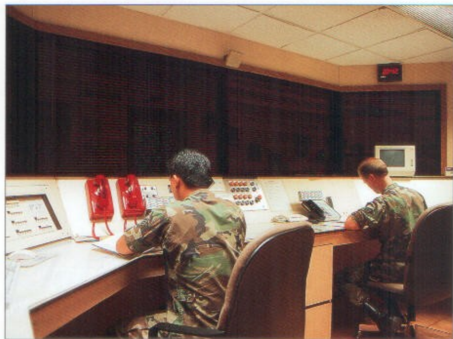
The communications control room should feature a state-of-the-art control console and ergonomically designed seating for personnel.
