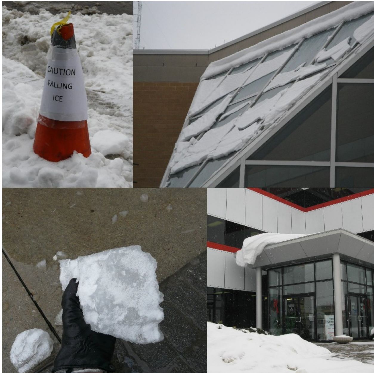
Examples of: Impromptu Caution Sign (upper left), Sliding Snow at Entry (upper right), Falling Ice from a Failed Snow Barrier (lower left), and Windblown Snow Cornice over Entry (lower right).
