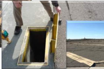
Unsecured Handhole at MCAS Beaufort
