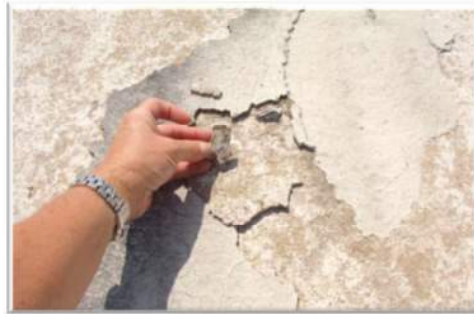
IPRF Figure 5-6. Heavy Paint Build Up on Concrete
