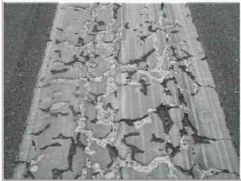
IPRF Figure 4-7. Many Layers of Paint on Asphalt
