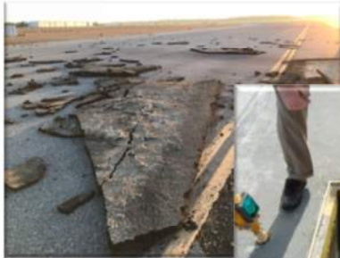
Blown out shoulder at NAS Patuxent River
