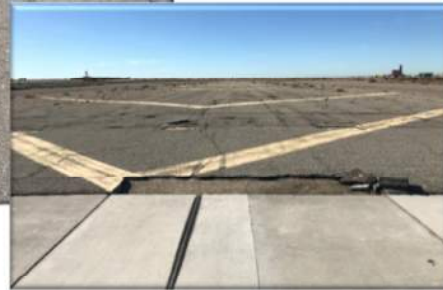
Blown out overrun at MCAS Yuma
