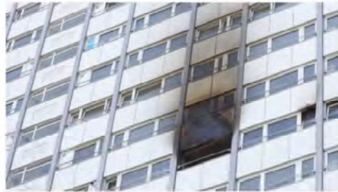
Smoke damage at Queensdale Crescent
