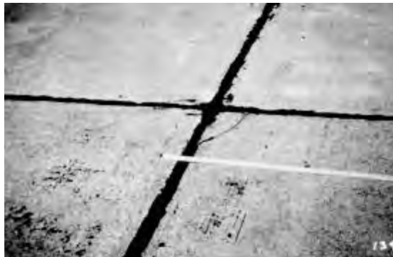
Figure 17.2. Low-severity corner spall
