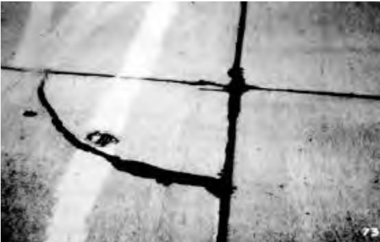
Figure 4.3. Low-severity corner break
