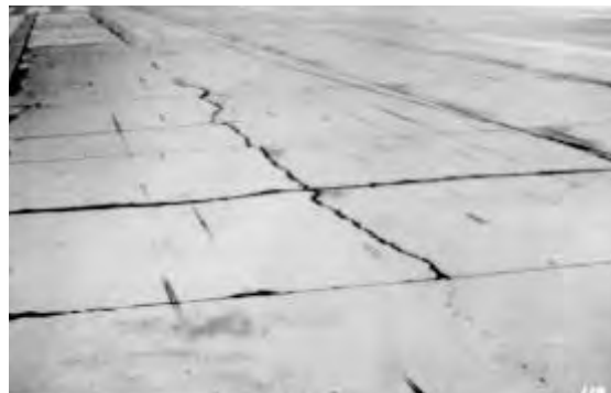
Figure 14.2. Low-severity intersecting cracks
