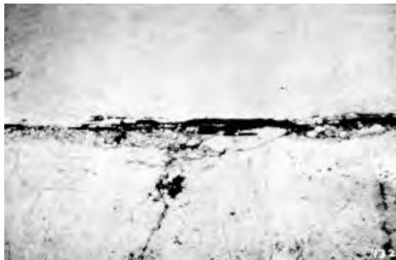
Figure 16.6. High-severity joint spall
