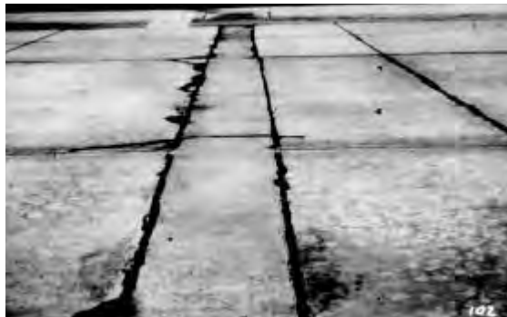
Figure 9.4. Low-severity utility cut
