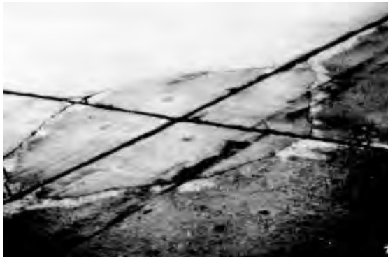
Figure 4.2. Low-severity corner break
