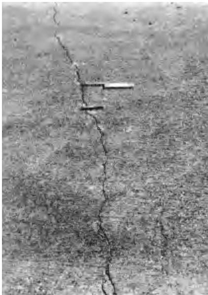
Figure 5.7. Medium-severity transverse crack
