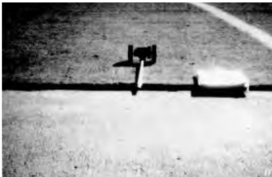
Figure 13.5. High-severity settlement on taxiway/runway, 3/4 in. (19.1 mm)
