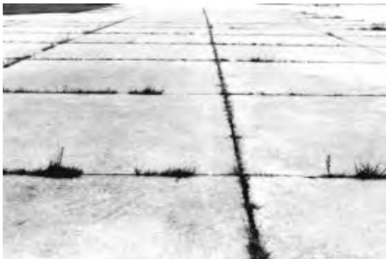
Figure 7.5. High-severity joint seal damage (extensive amount of weed growth)
