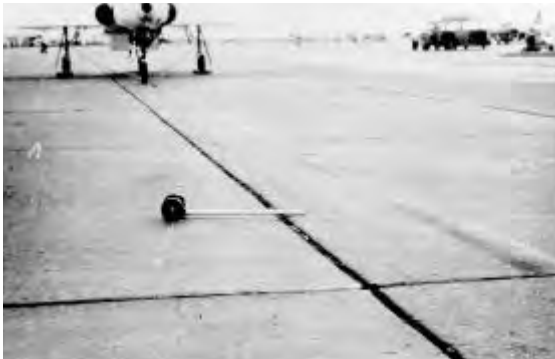
Figure 13.3. Low-severity settlement on apron
