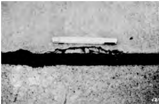
Figure 16.3. Low-severity joint spall
