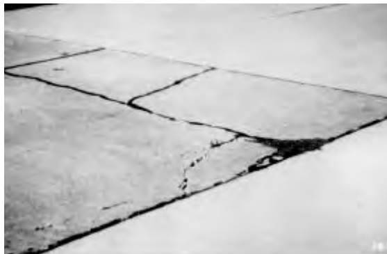
Figure 14.4. Medium-severity intersecting cracks
