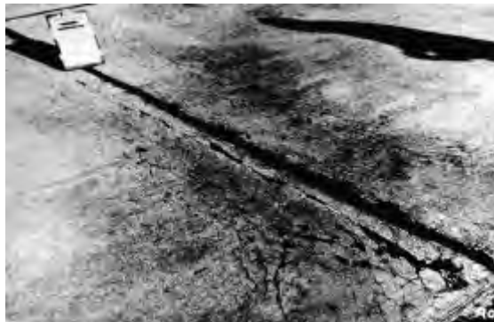
Figure 6.6. High-severity “D” cracking (the “D” cracking occurs over more than one joint with some disintegration)
