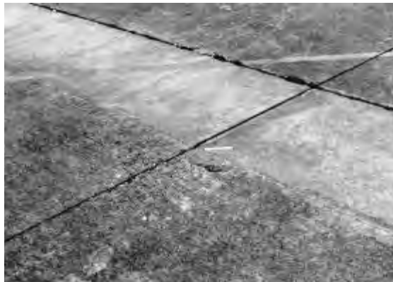
Figure 6.2. Low-severity "D" cracking
