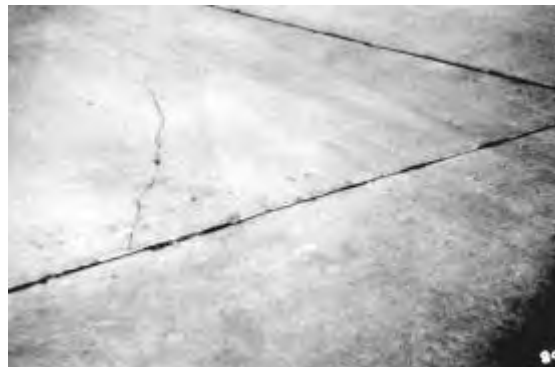
Figure 5.4. Low-severity diagonal crack
