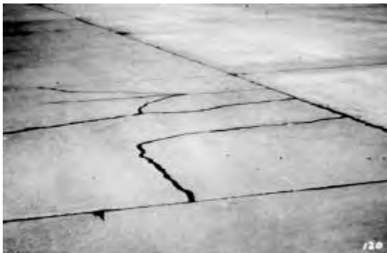
Figure 14.3. Low-severity intersecting cracks
