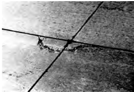
Figure 17.6. High-severity corner spall
