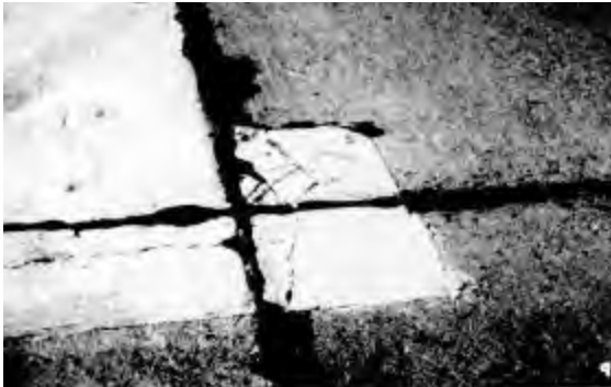
Figure 8.5. Medium-severity small patch
