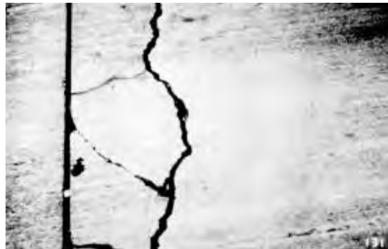
Figure 16.4. Medium-severity joint spall
