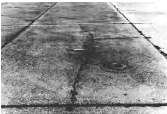
Figure 5.9. High-severity longitudinal cracks
