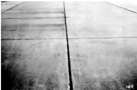
Figure 11.3. Pumping (note stains on pavement)
