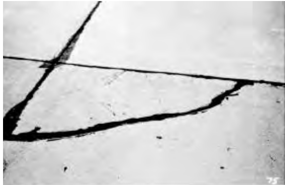
Figure 4.4. Medium-severity corner break (area between the corner break and the joints is lightly cracked)
