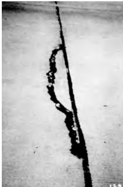
Figure 16.2. Low-severity joint spall
