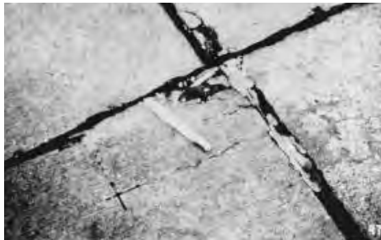
Figure 8.4. Medium-severity small patch
