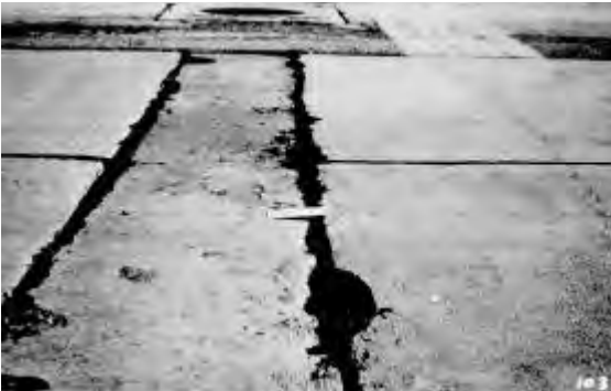
Figure 9.5. Medium-severity utility cut
