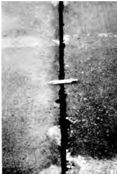
Figure 7.2. Low-severity joint seal damage
