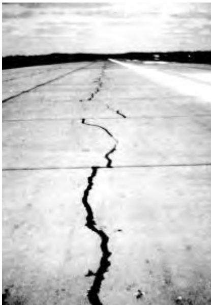
Figure 5.3. Low-severity longitudinal crack
