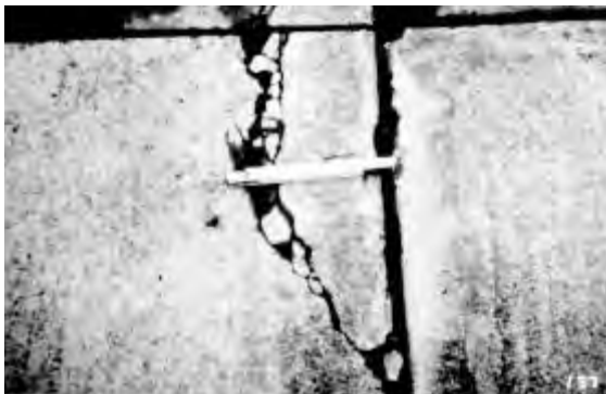
Figure 17.5. Medium-severity corner spall
