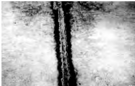
Figure 11.4. Pumping (close-up of fine materials collecting in the joint)
