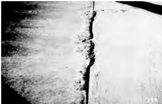
Figure 16.7. High-severity joint spall
