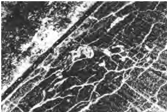
Figure 6.5. Medium-severity “D” cracking occurring in limited area of slab
