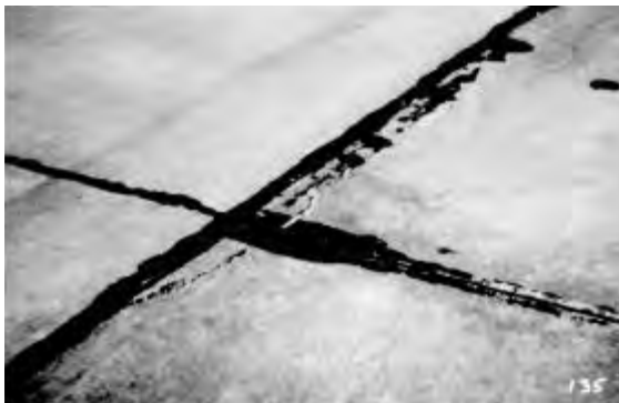
Figure 17.3. Low-severity corner spall
