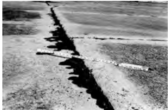
Figure 13.4. Medium-severity settlement on apron >1/2 in. (>12.7 mm)
