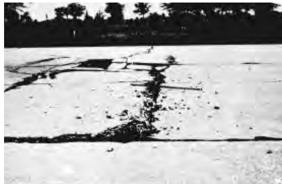
Figure 3.2. Low-severity blowup (note that this would only be considered low severity if the shattering in the foreground were the only part existing and the foreign material were removed)
