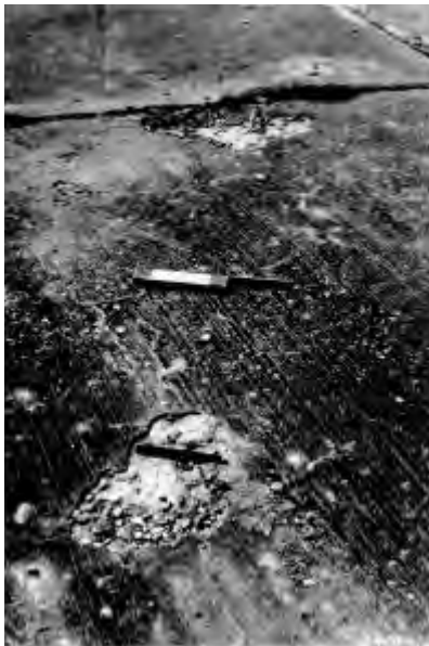
Figure 12.5. Close-up of high-severity scaling
