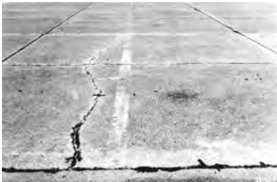
Figure 5.5. Medium-severity longitudinal crack
