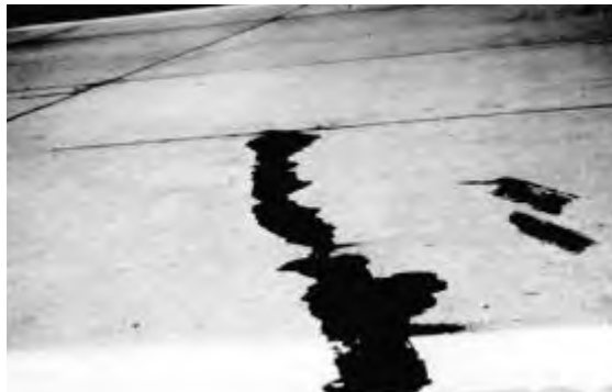
Figure 5.6. Medium-severity transverse crack
