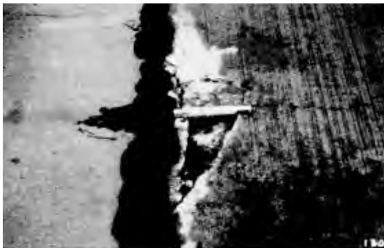
Figure 16.5. Medium-severity joint spall
