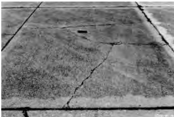
Figure 14.5. Medium-severity intersecting cracks
