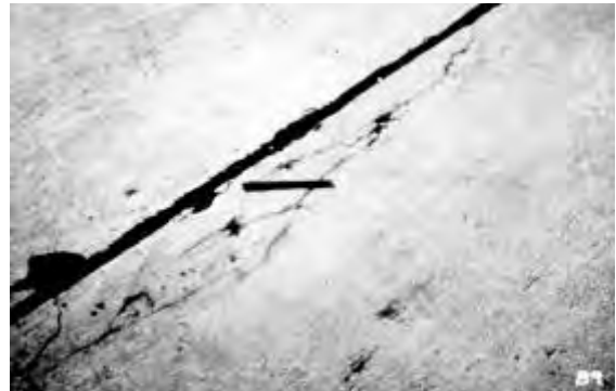
Figure 6.4. Medium-severity "D" cracking
