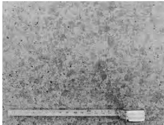
Figure 12.6. High-severity scaling caused by alkali aggregate reaction. This could be low- or medium-severity alkali-silica reaction, depending on the extent of coverage over the slab
