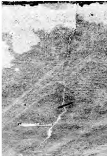
Figure 5.2. Low-severity longitudinal crack
