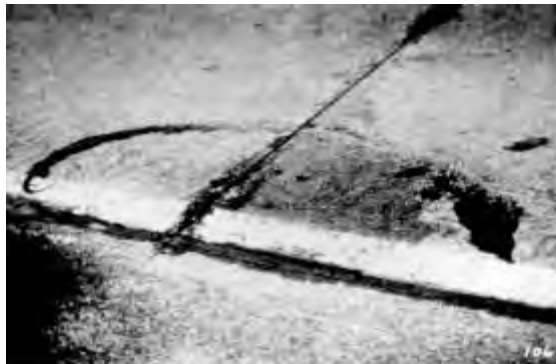
Figure 11.2. Pumping (note fine material on surface that has been pumped and has caused corner break)
