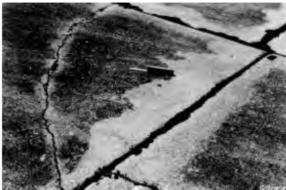
Figure 4.5. Medium-severity corner break
