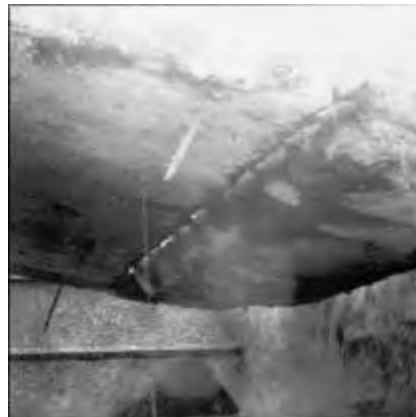
Figure 4.2. Bottom of deteriorated slab
