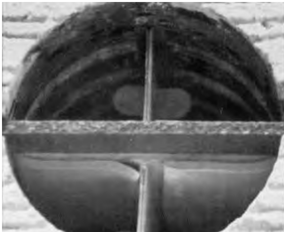
Figure 10.3. Core hole centered over crack
