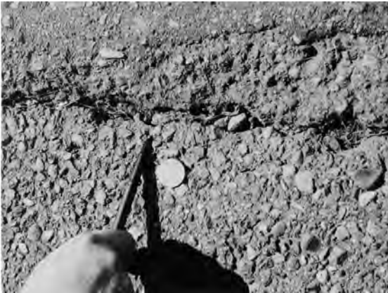
Figure 7.3. Example of a medium-size crack
