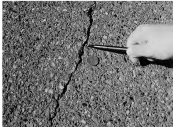
Figure 7.2. Example of a small-size crack
