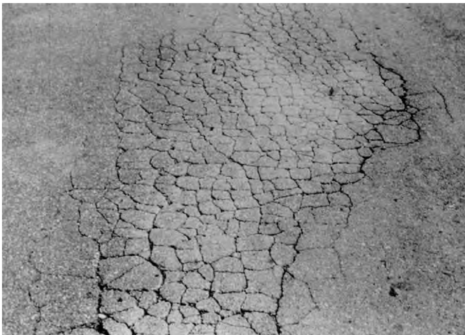
Figure 2.1. Example of alligator cracking
