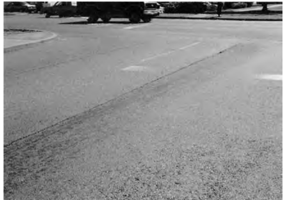
Figure 3.2. Example of longitudinal cracking
