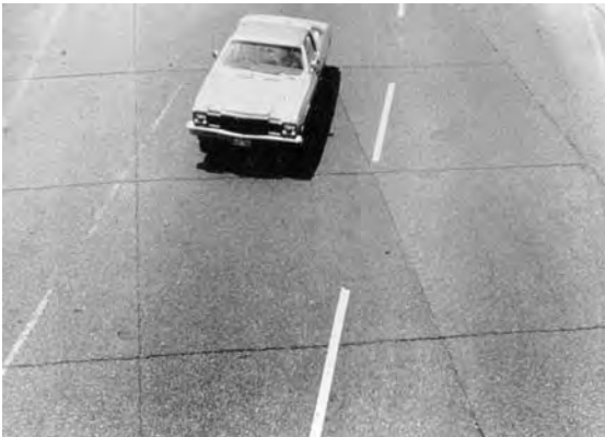
Figure 3.1. Example of reflective cracking
