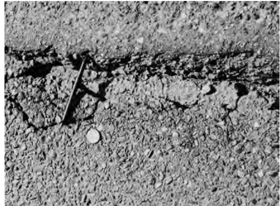
Figure 7.4. Example of large-size crack
