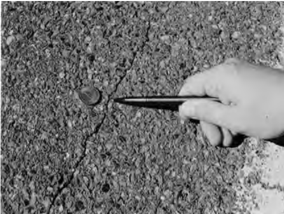
Figure 7.1. Example of hairline-size crack
