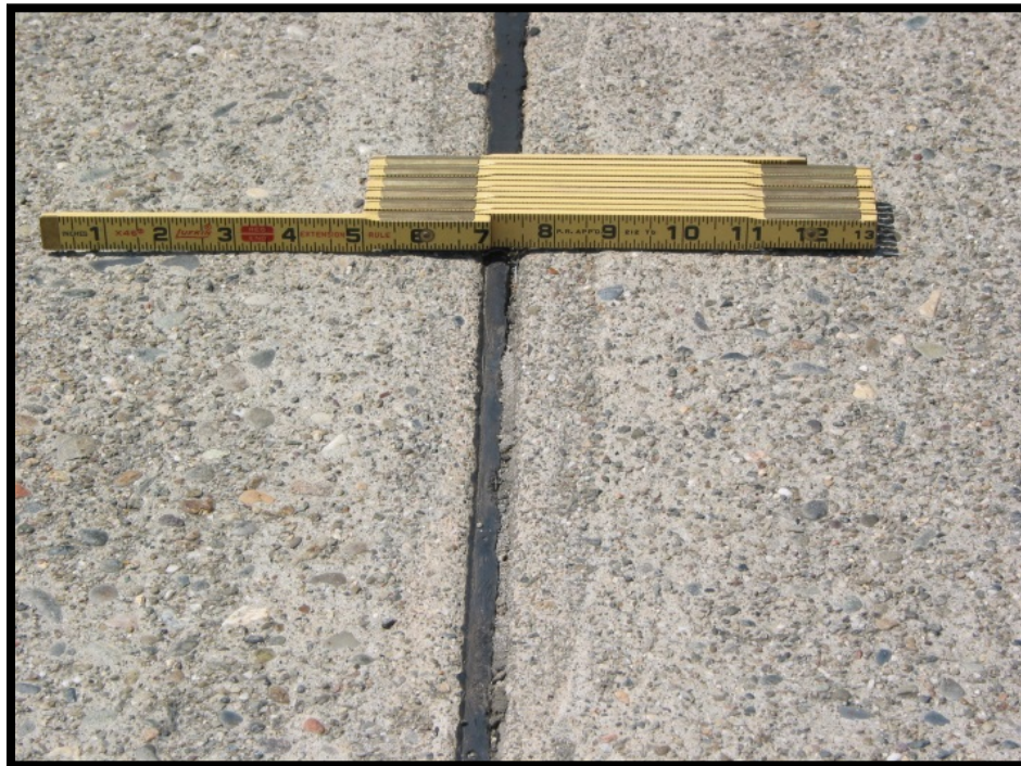
Figure B-15 Low-Severity Joint Seal Damage
