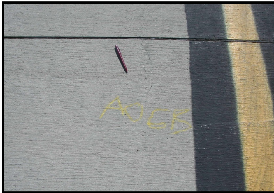
Figure B-36 Shrinkage Cracks
