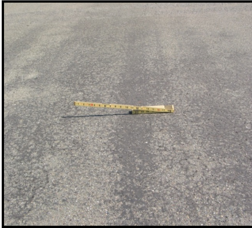
Figure A-5 Bleeding
