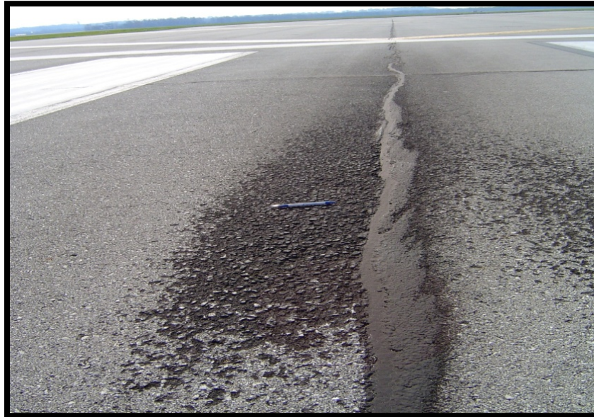
Figure A-20 Jet Blast Erosion
