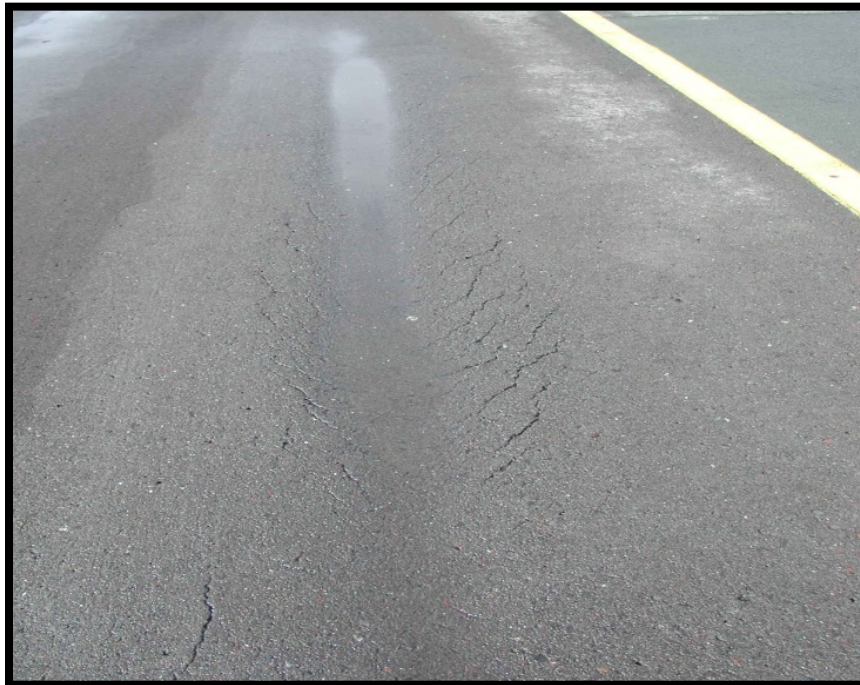
Figure A-46 Rutting
