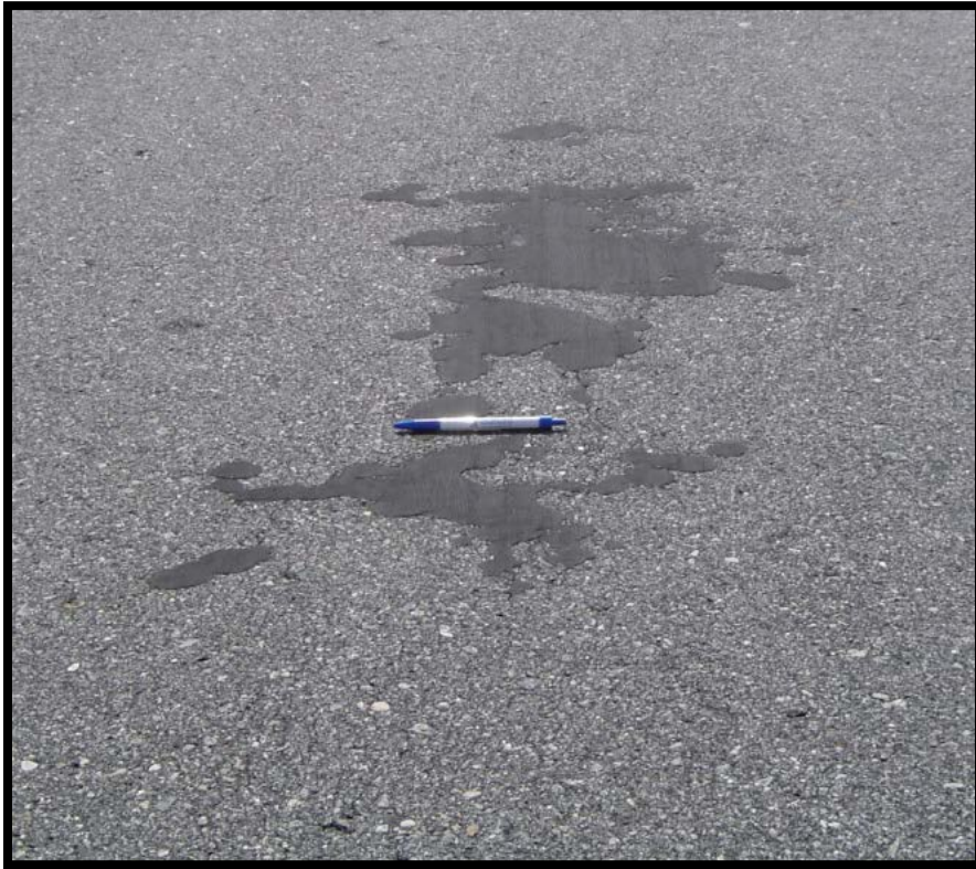
Figure A-4 Bleeding
