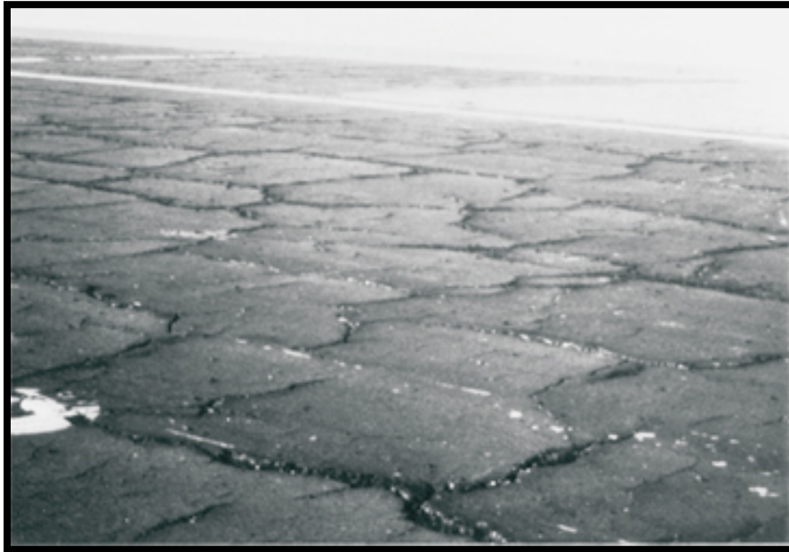
Figure A-11 High-Severity Block Cracking
