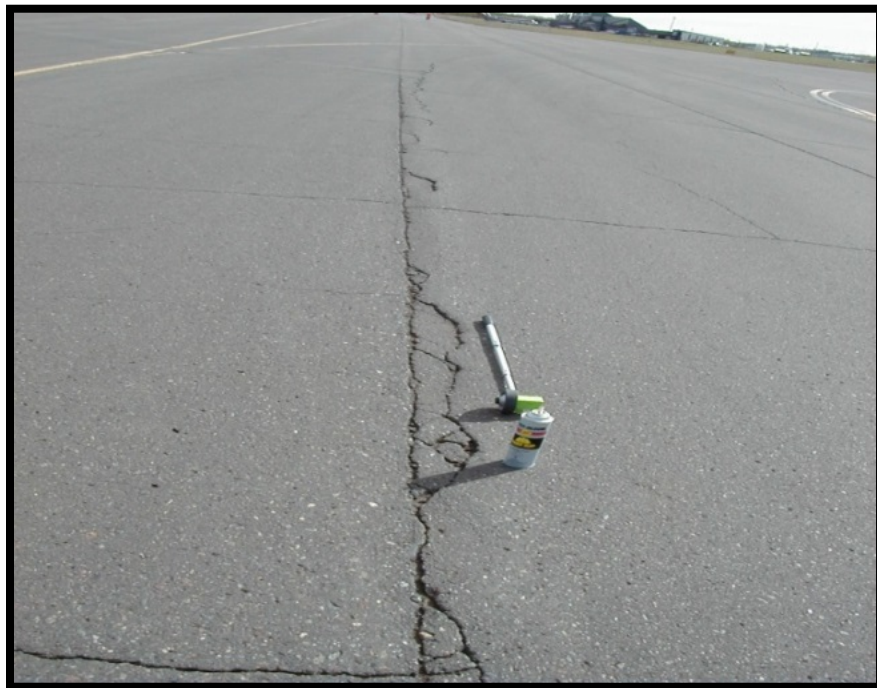
Figure A-23 High-Severity Joint Reflection Cracking
