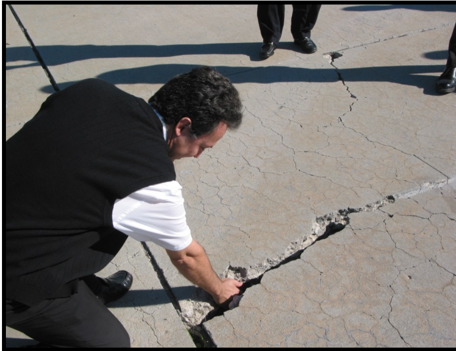
Figure B-46 High-Severity ASR
