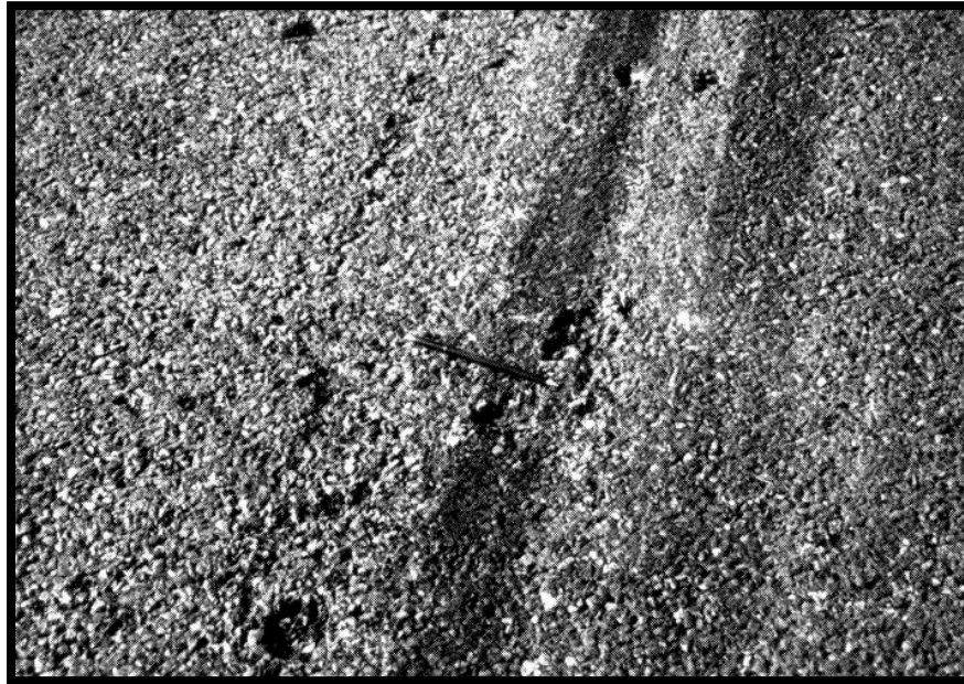
Figure A-45 High-Severity Raveling (PFC)
