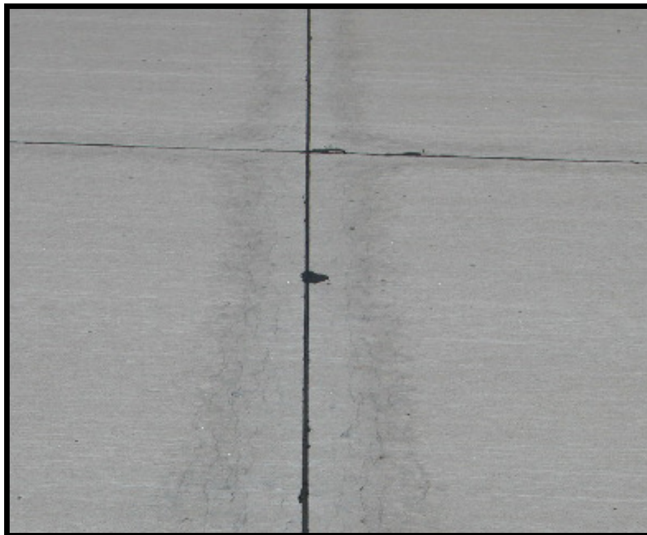
Figure B-12 Low-Severity “D” Cracking
