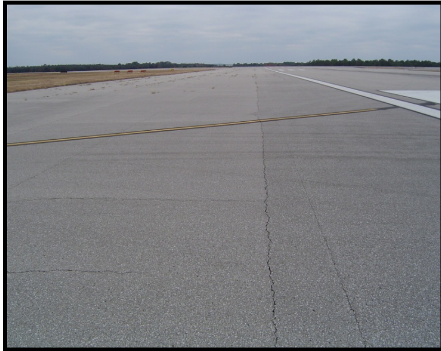
Figure A-22 Medium-Severity Joint Reflection Cracking
