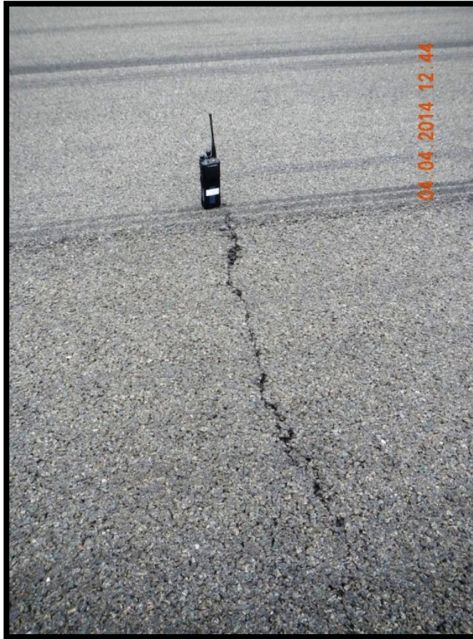
Figure A-29 Medium-Severity PFC L&T Cracking
