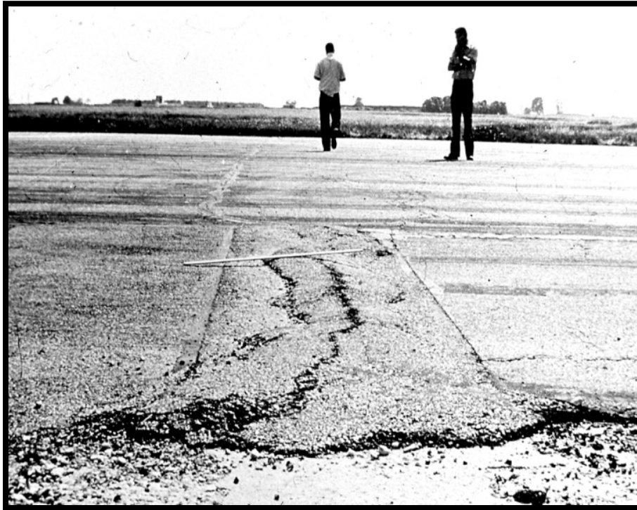
Figure A-34 High-Severity Patching
