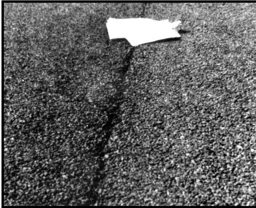
Figure A-30 High-Severity PFC L&T Cracking
