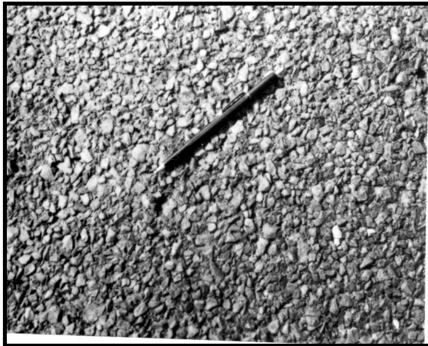
Figure A-42 Low-Severity Raveling (PFC)
