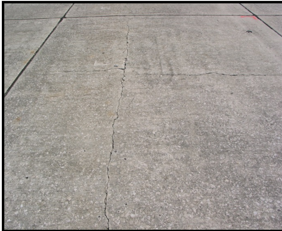
Figure B-33 Low-Severity Shattered Slab/Intersecting Cracks
