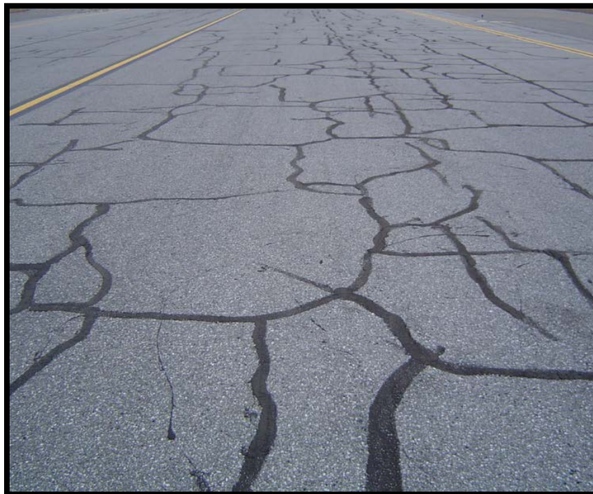
Figure A-6 Low-Severity Block Cracking
