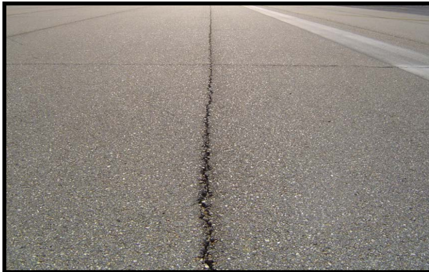
Figure A-21 Low-Severity Joint Reflection Cracking
