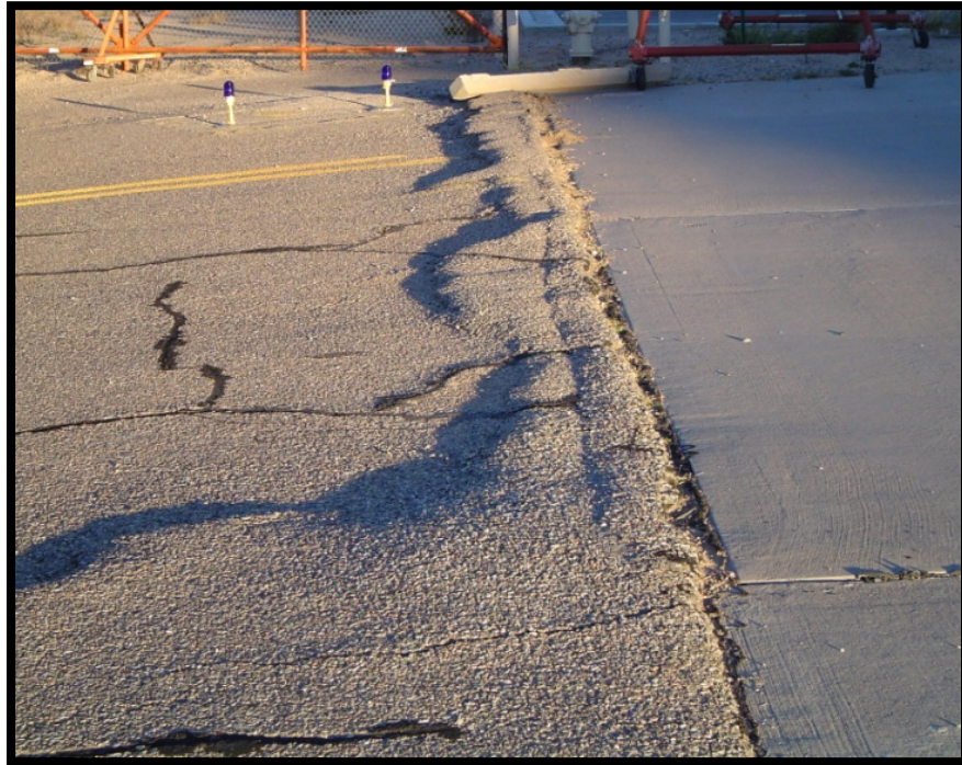
Figure A-49 High-Severity Shoving
