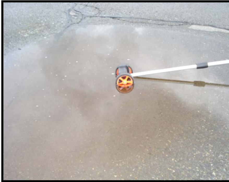
Figure A-19 High-Severity Depression
