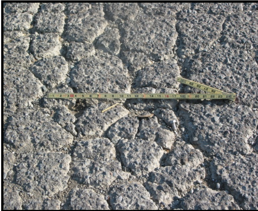
Figure A-3 High-Severity Alligator Cracking
