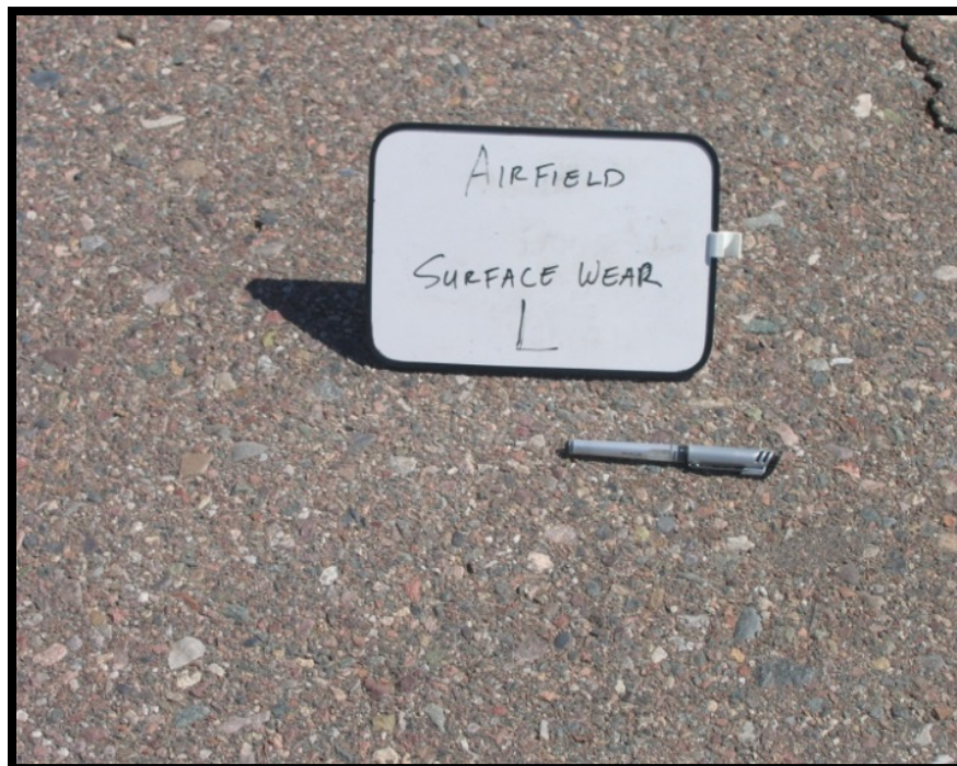
Figure A-54 Low-Severity Weathering
