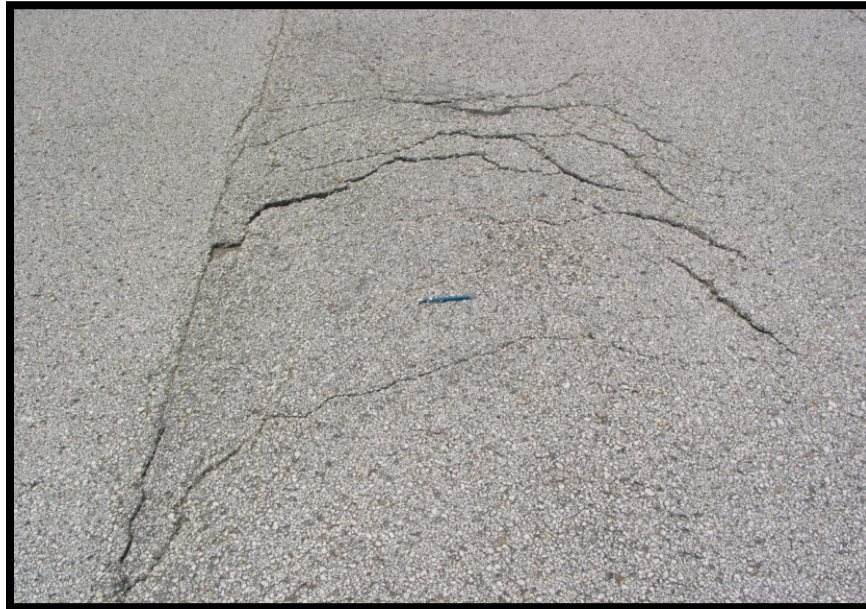
Figure A-50 Slippage Cracking
