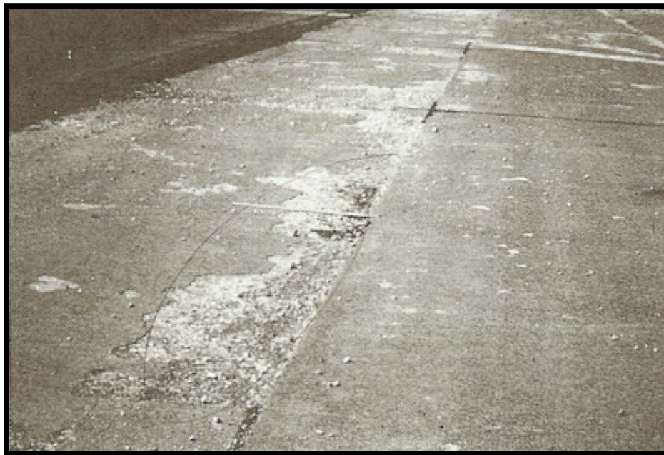
Figure B-29 High-Severity Scaling
