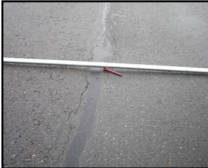
Figure A-16 Low-Severity Depression
