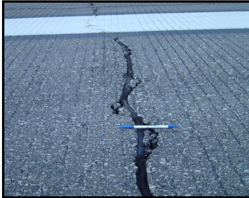
Figure A-26 High-Severity L&T Cracking
