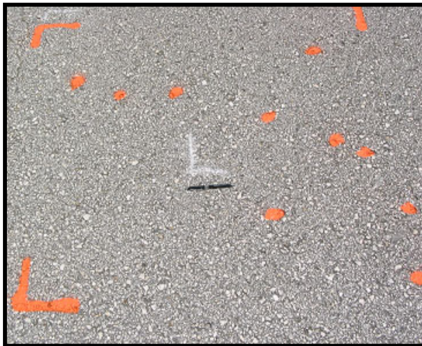
Figure A-36 Low-Severity Raveling (Dense Mix)
