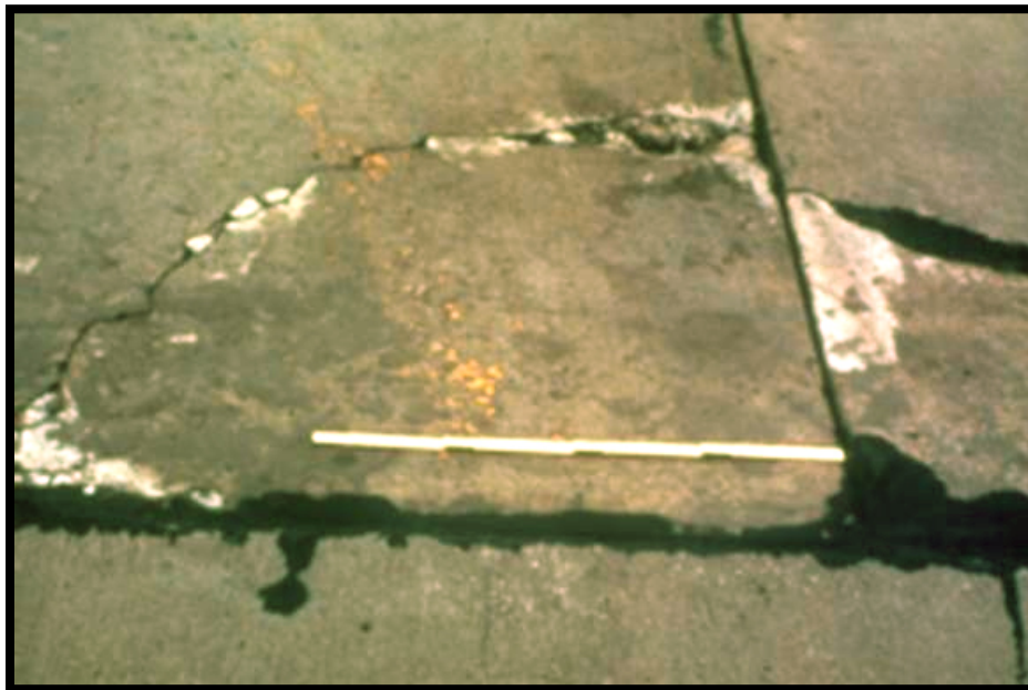
Figure B-7 High-Severity Corner Break
