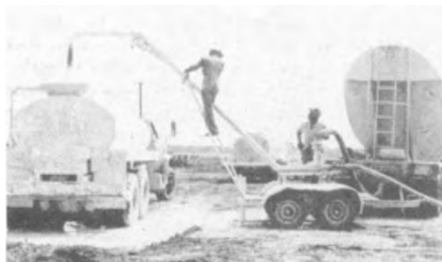
Figure 4-30. Jet slurry mixing plant.
