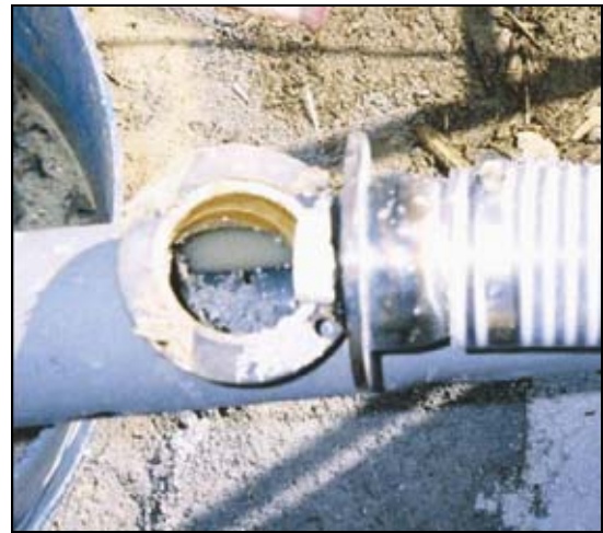
Figure A-15. Flex hose connection.
