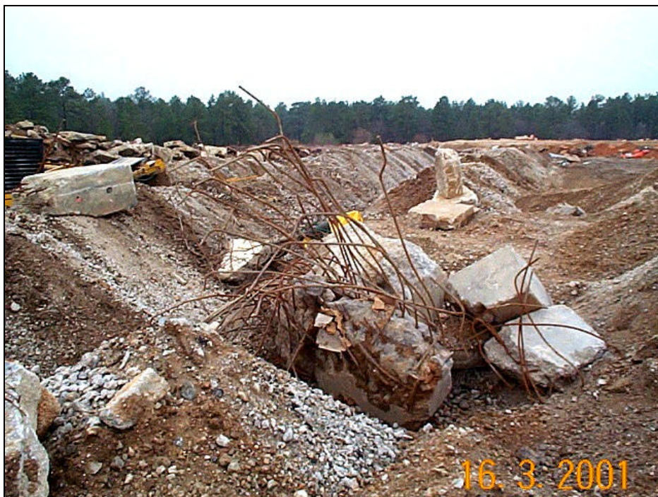
Figure 12. When a Road or Structure Is Demolished, the Rebar can Often Be Seen Protruding from the Broken Chunks of Portland Cement Concrete.
