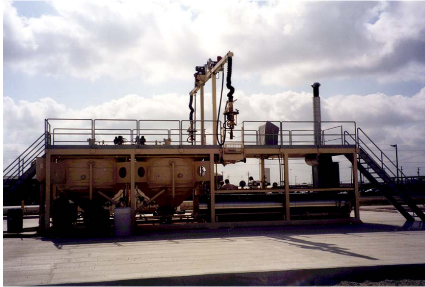
Figure 5 – Off-the-shelf purging system at Fort Hood, TX
