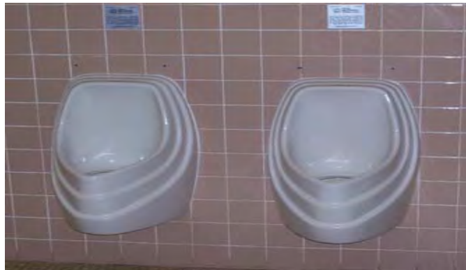
Figure A-25. Waterless urinals installed at Fort Huachuca (Scholze 2010).
