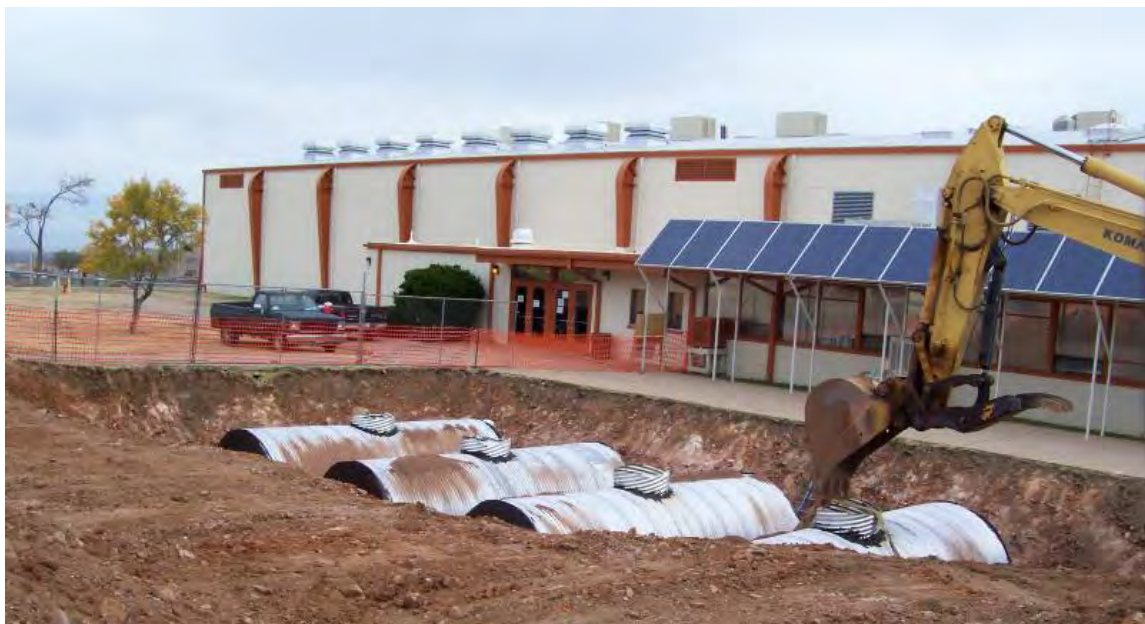
Figure A-21. Capture of rainwater for infiltration purposes at Fort Huachuca (Courtesy of Tom Runyon, Fort Huachuca).
