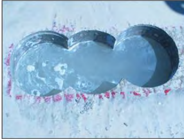
Figure 17. Three Adjacent 12-Inch (0.3-m) Cores Allow for Insertion of the Hat-Type Tie-Down.
