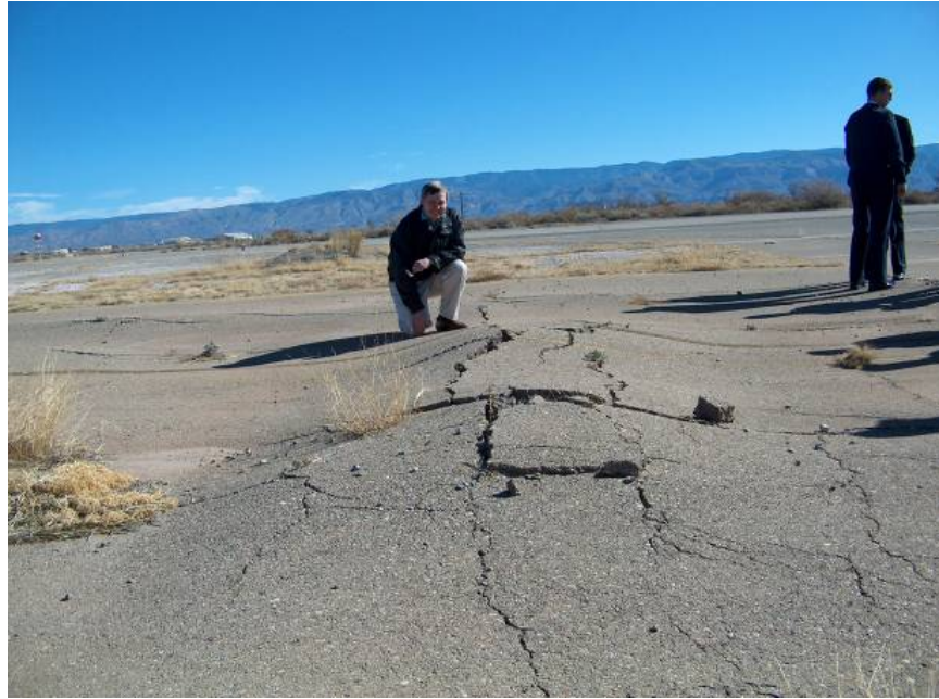
Figure 2. Example of Localized Heaving in a Flexible Pavement Caused by Volume Change in the Underlying Base Course
