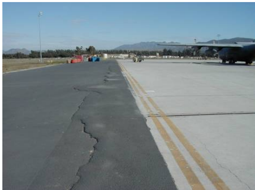
Figure 5. Examples of Damage to Adjacent Asphalt from ASR-Induced Expansion in Adjacent PCC Pavement. This suggests of a highly reactive pavement.
