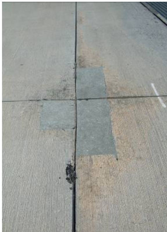
Figure 4. Minor ASR Cracking in 5-Year-Old Pavement (Left Photograph); Patching Needed 3 Years Later (Right Photograph). Because of the early development of ASR symptoms in this Holloman AFB pavement, it would be considered a highly reactive pavement.
