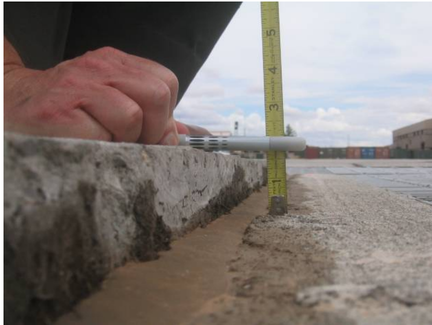
Figure 1. Example of Differential Heaving on a Rigid Pavement Caused by Volume Change in Underlying Base and Fill Layers
