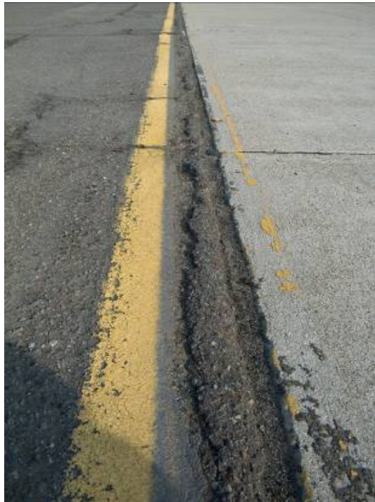
Figure 7. Example of Low Reactivity ASR at Travis AFB. Cracking is generally tight, with minor FOD issues in this pavement that is over 25 years old. Small volume change has caused minor upheaving of the AC shoulder. The only maintenance on this ramp has been sweeping to minimize the hazard cause by the slow generation of FOD.
