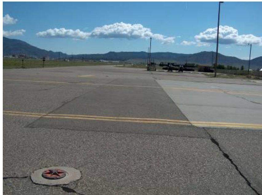
Figure 6. Examples of Large Volume Changes Suggesting Highly Reactive ASR Pavements. On the left, two pavement slabs are displaced by several inches. On the right, the PCC has grown from the visible joint in the AC and damaged the adjacent pavement. An AC repair patch to the damaged AC from this growth is visible to the left of the PCC.
