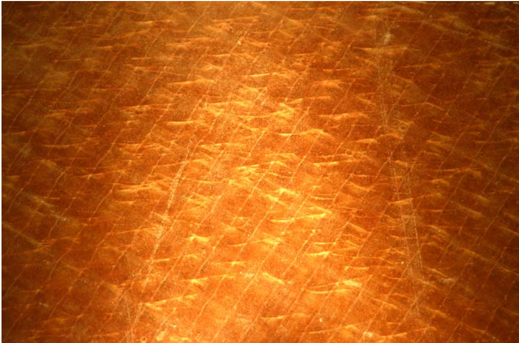
Figure 2. Unidirectional Cracking Seen with Angled Flashlight
