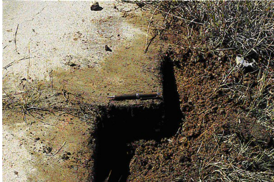
Figure 7. Misalignment of Slabs Caused by Differential ASR Expansion, Kirtland AFB.
