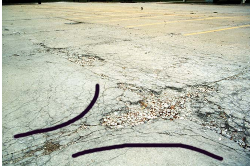
Figure 6. D-cracking at Grissom AFB (Not to be Confused with ASR-induced Cracking). Note general C-shape of cracks that are roughly asymptotic to joints and that do not cross transverse joints as seen in Figures 2 and 3.
