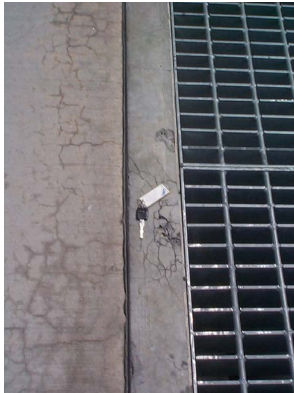
Figure 9. Trench Drain Damage from ASR Expansion, Holloman AFB.
