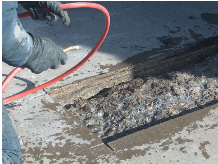
Figure 11. ASR Gel—Appearing as Light, Hazy Coating on Shallow Patching Repairs at Holloman AFB—Was Impossible to Remove and Caused Many Patch Bond Failures.
