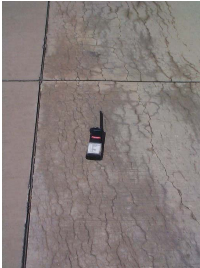
Figure 2. ASR-induced Cracking on Taxiway, Holloman AFB. Note cracks are preferentially longitudinal and continue across transverse joints.
