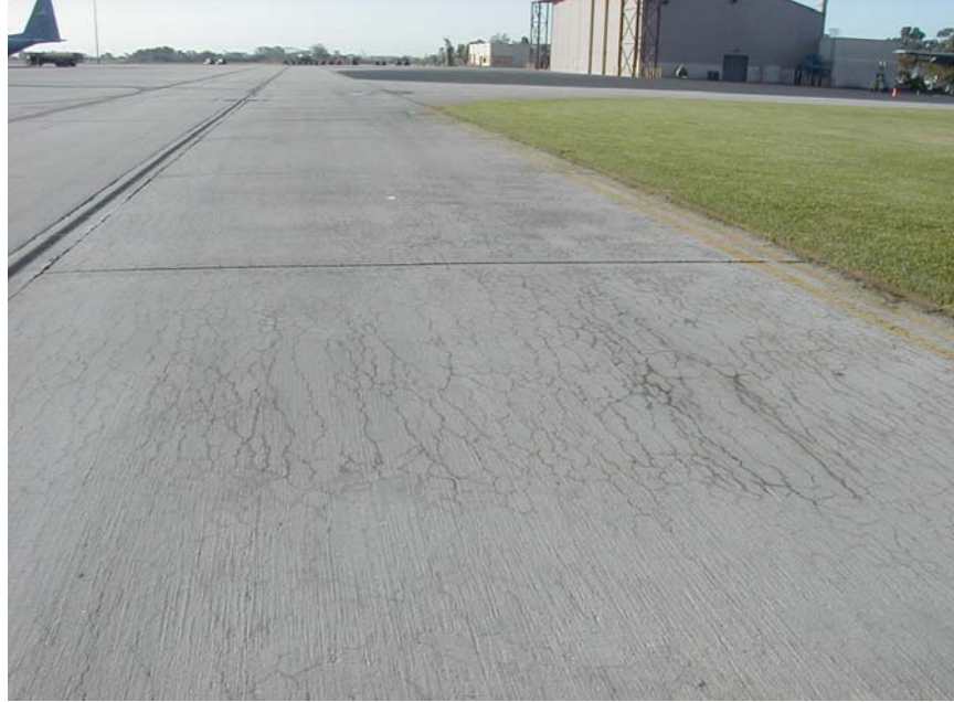
Figure 3. ASR-induced Cracking in Taxiway at Channel Island ANG Facility. Note cracks are preferentially longitudinal and continue across transverse joints.
