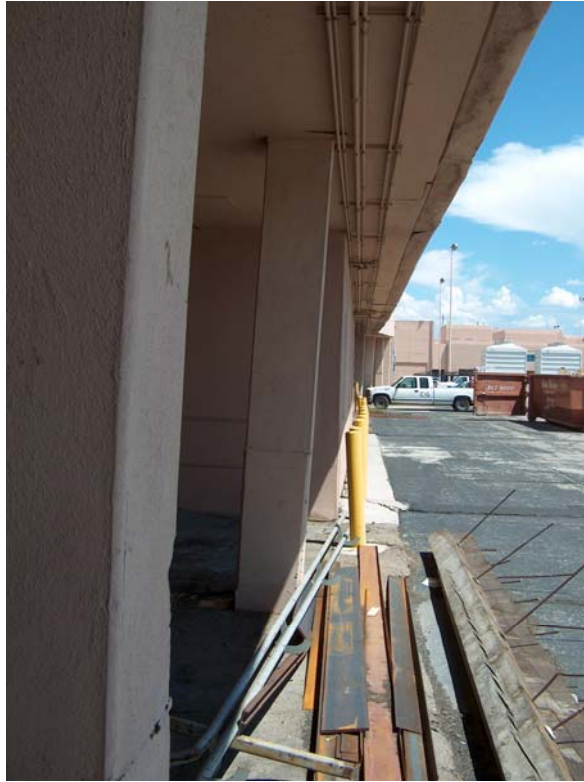
Figure 10. Building Column Pushed out of Alignment by ASR Volume Expansion in Adjacent Concrete Pavement, Albuquerque, NM.
