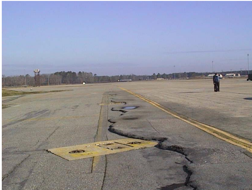
Figure 8. Asphalt Shoulder Heaving Caused by ASR Expansion in Adjacent Concrete at Seymour-Johnson AFB.
