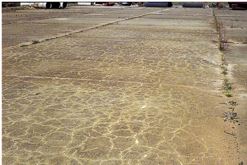
Figure 4. ASR-induced Cracking in Ramp at Tinker AFB. Note cracks are random (without the preferential longitudinal orientation seen in Figures 1 and 2) and continue across joints.
