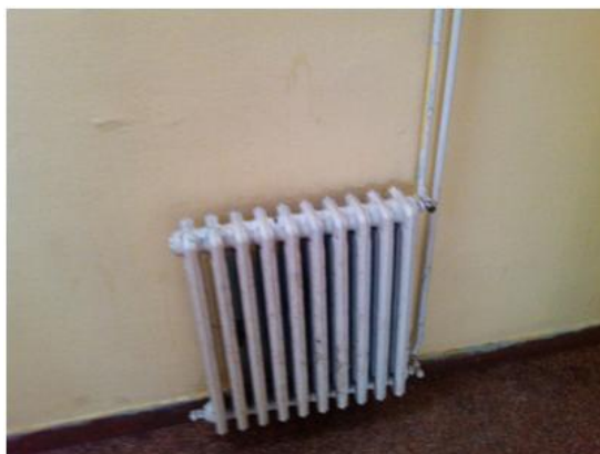
Source: Fichtner Figure G-52. Typical existing radiator in corridors.
