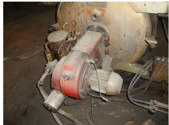
Source: Fichtner Figure G-51. Burner on old boiler.
