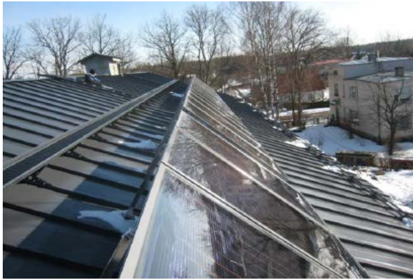
Figure C-9. Installed solar thermal system.
