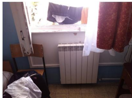
Source: Fichtner Figure G-53. Typical "new" radiator in the rooms.
