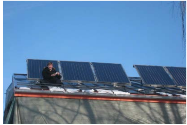
Figure C-10. Installed solar thermal system.
