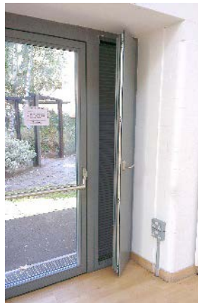
Figure I-14. Manual air intake panel for secure night-purge ventilation.
