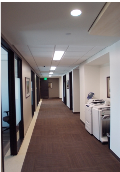
Figure J-57. LED lighting OPM space.
