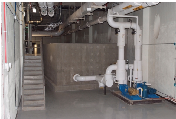
Figure J-64. Water storage tank.
