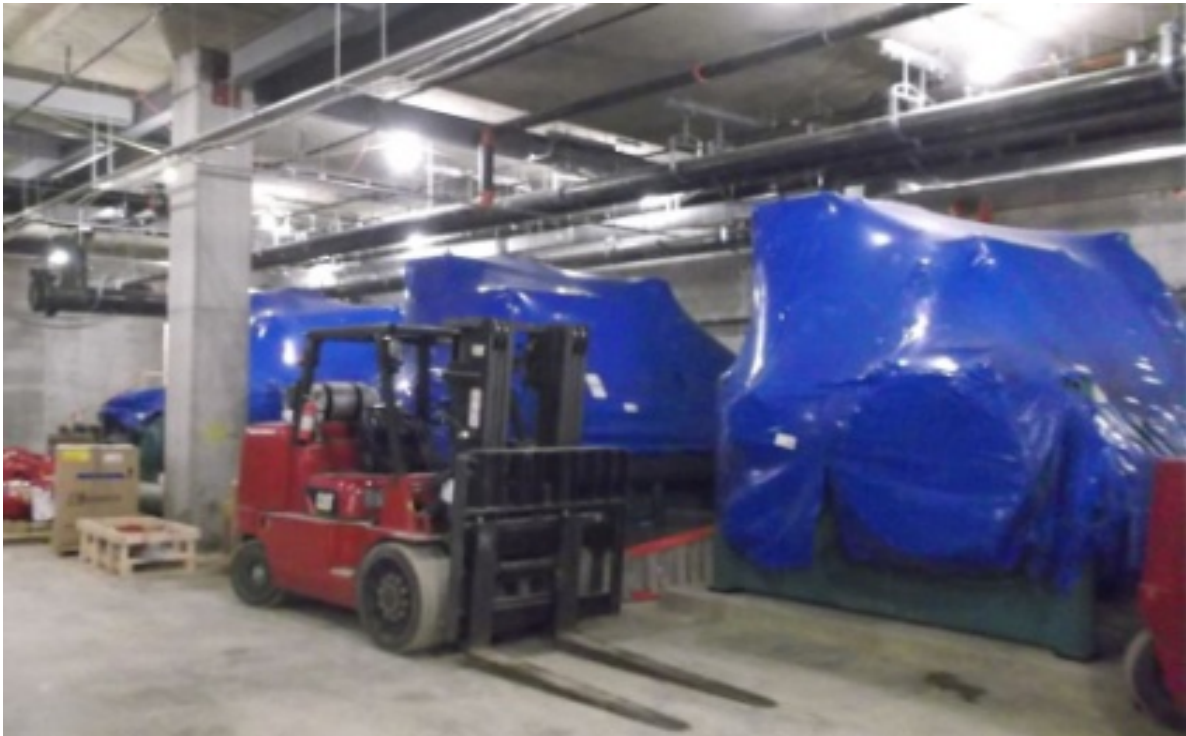
Figure J-27. CMP chillers.
