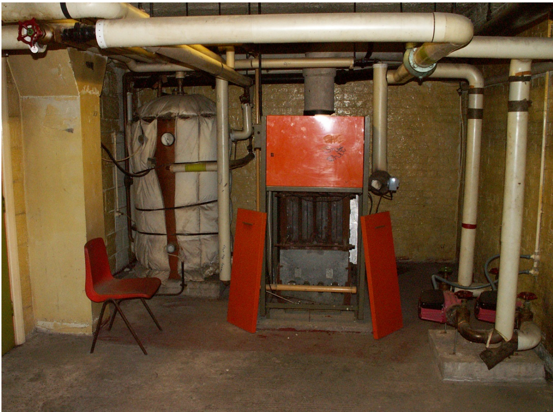
Figure I-5. Before retrofit: Boiler room,
