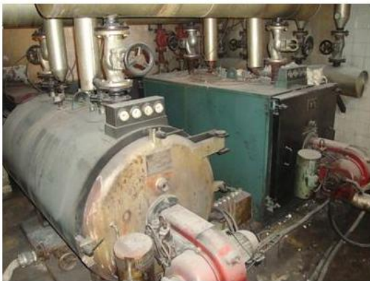
Source: Fichtner Figure G-50. Boilers "TKT Toplota Zagreb."
