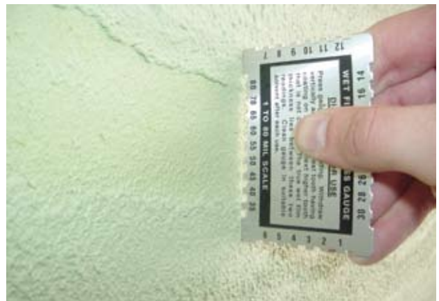
ABAA Certified Installers Daily Quality Control. Thickness testing of a liquid applied air barrier.
