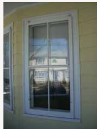
A traditional wood storm window fastened by hangers at the top. This storm window is also secured by four screws along the perimeter.
